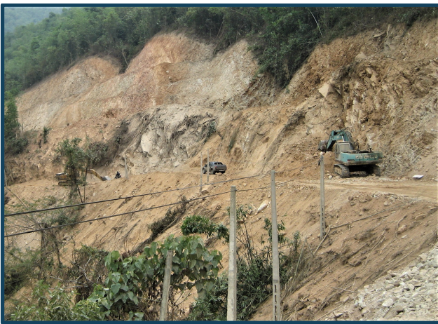
Earthworks without drainage or support prior to monsoon season, Vietnam.
