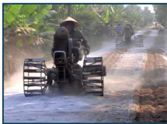
Use of agricultural machinery in mixing of lime and local soil for LVRR stabilised base layer. Photo J Cook
