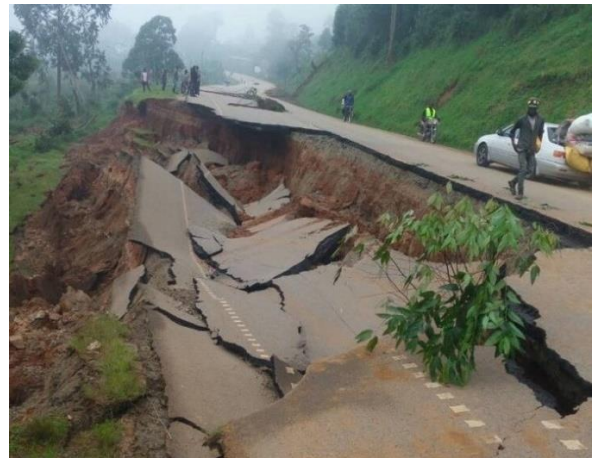
5B Fill slope failure with underlying soft clay
