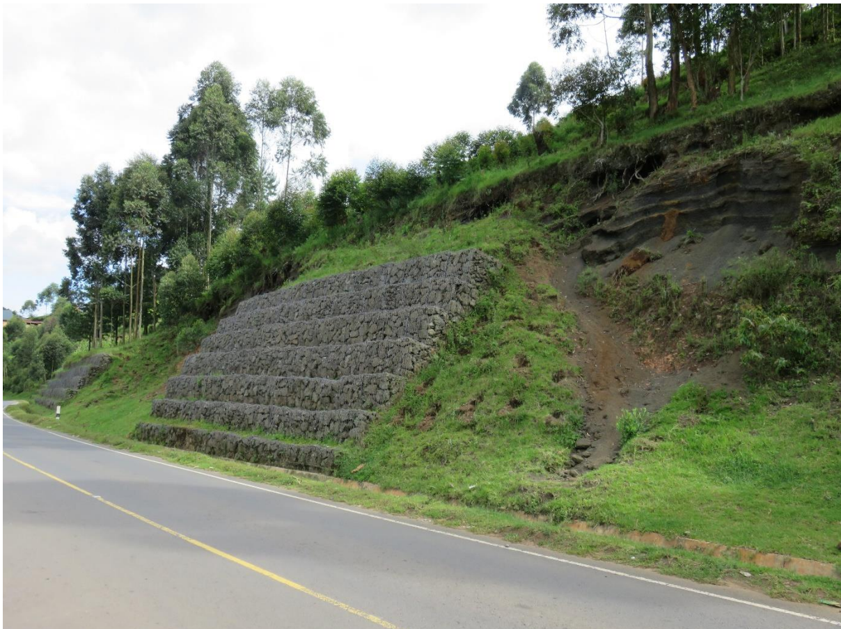
Figure 7 - Use of gabion retaining walls to support vulnerable sections of cut slope
