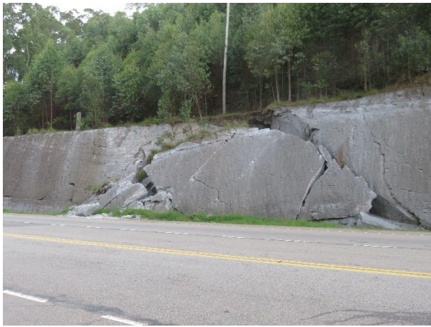
5A Rock failure along adverse joints
