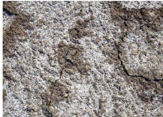
Figure 4-15: Salt deposition on the soil surface
