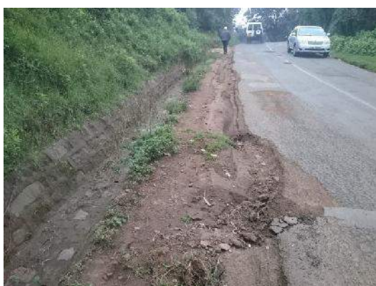
Figure 9-18: Poor – Gap between surfacing and drain lining
