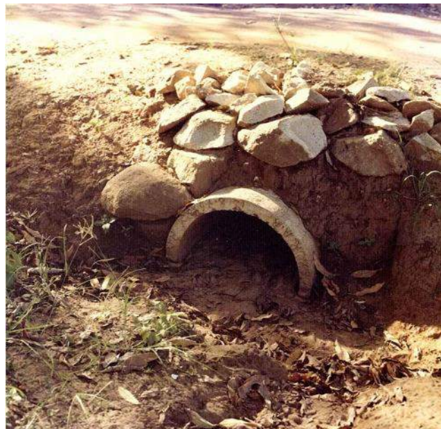
Figure 8-25: Siltation problems at culvert outlet
