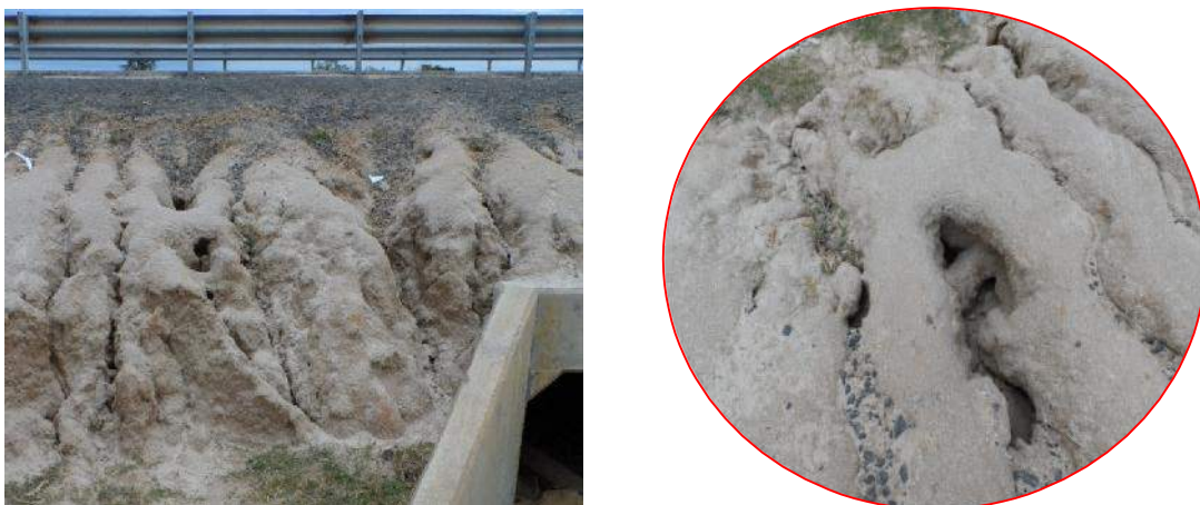
Figure 4-12: Piping in dispersive soils
