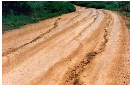
Longitudinal erosion in fine material
