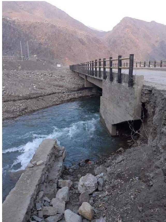
Figure 4-24: Typical bridge scour
