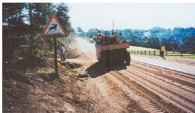
Figure 12-6: Extensive rolling of an Otta Seal is essential to achieve a good result
