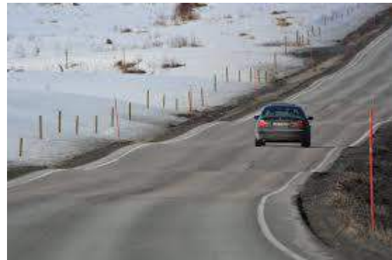
Figure 10-14: Pavement affected by frost heave
