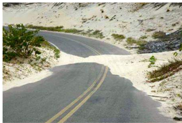
Figure 4-30: Road safety risk caused by sand on roadway
