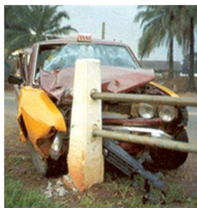
Badly designed bridge railing
