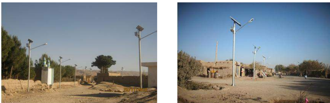
Figure 4-22: LED solar powered street lighting in Afghan villages
