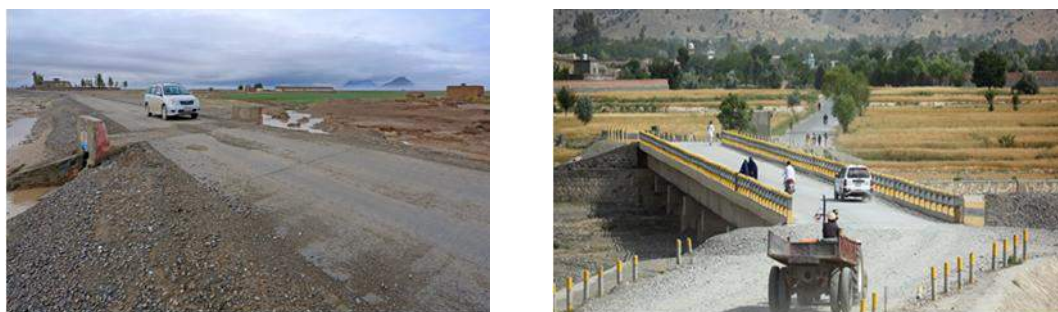
Figure 4-25: Road safety challenges at culverts and narrow bridge structures
