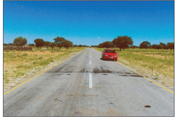
Figure B.9.15: Example of poor transverse joint construction
