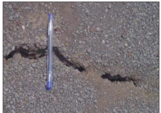
Figure B.4.7: Longitudinal cracking and deformation due to an expansive subgrade
