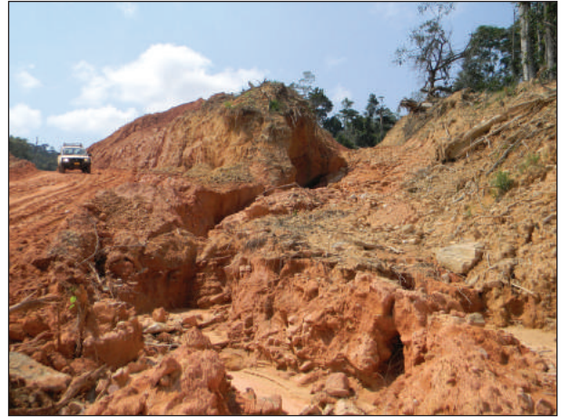
Figure B.4.14: Example of severe erosion in erodible/dispersive soils
