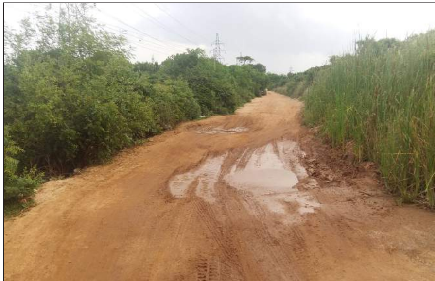
Figure C.9.2: Stagnant water due to poor camber
