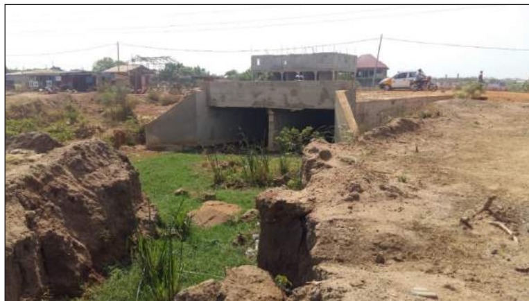
Figure C.6.7: Erosion of channel downstream of culvert
