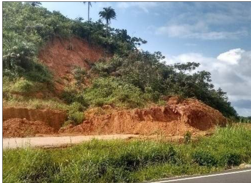
Figure C.7.4: Slope failure in weathered mantle
