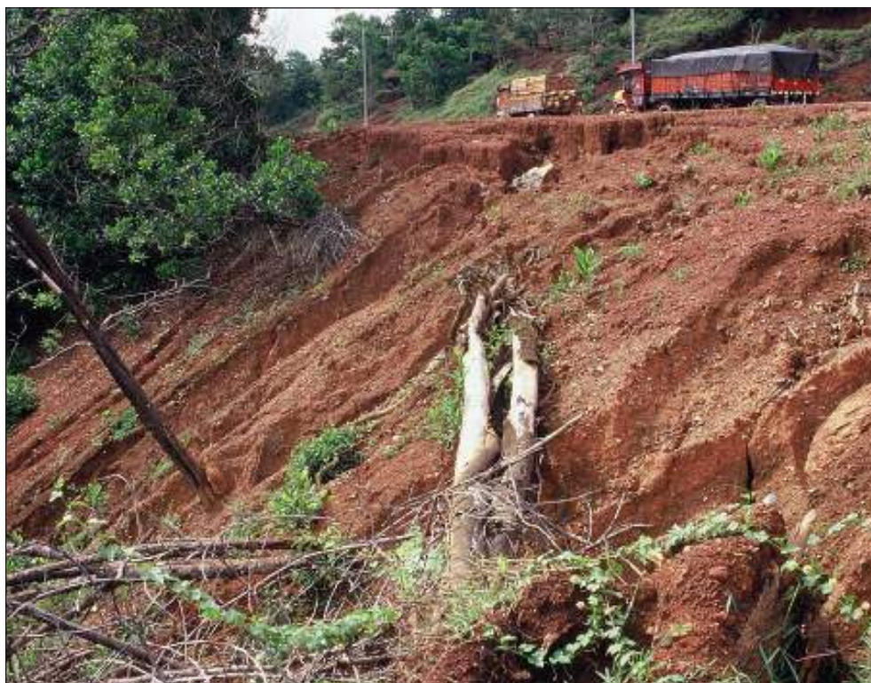
Figure C.7.12: Severe erosion of embankment material
