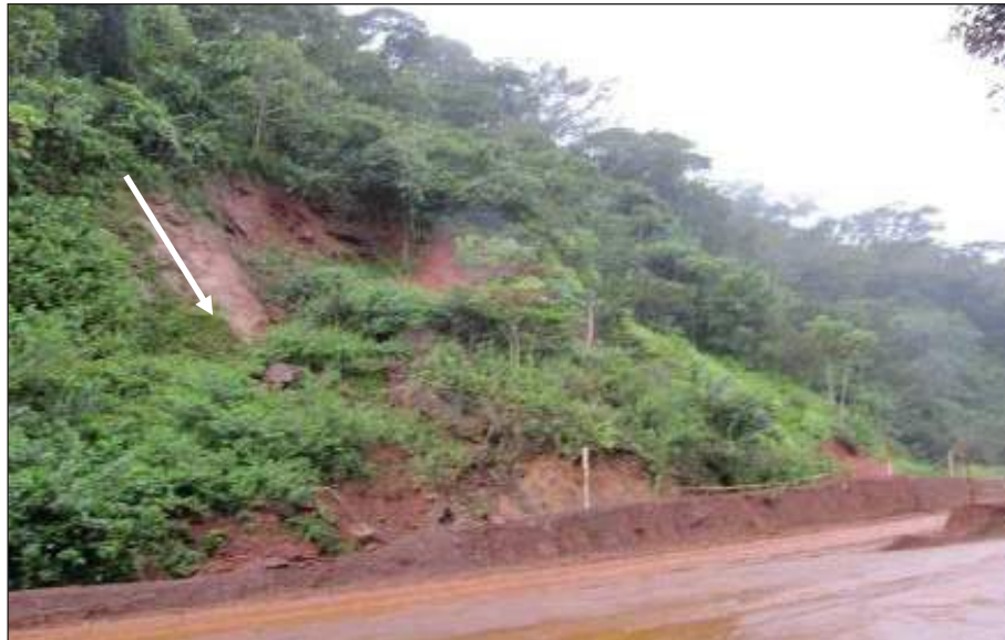
Figure C.7.1: Slope failure along adverse rock joints (arrow indicates joint surface)
