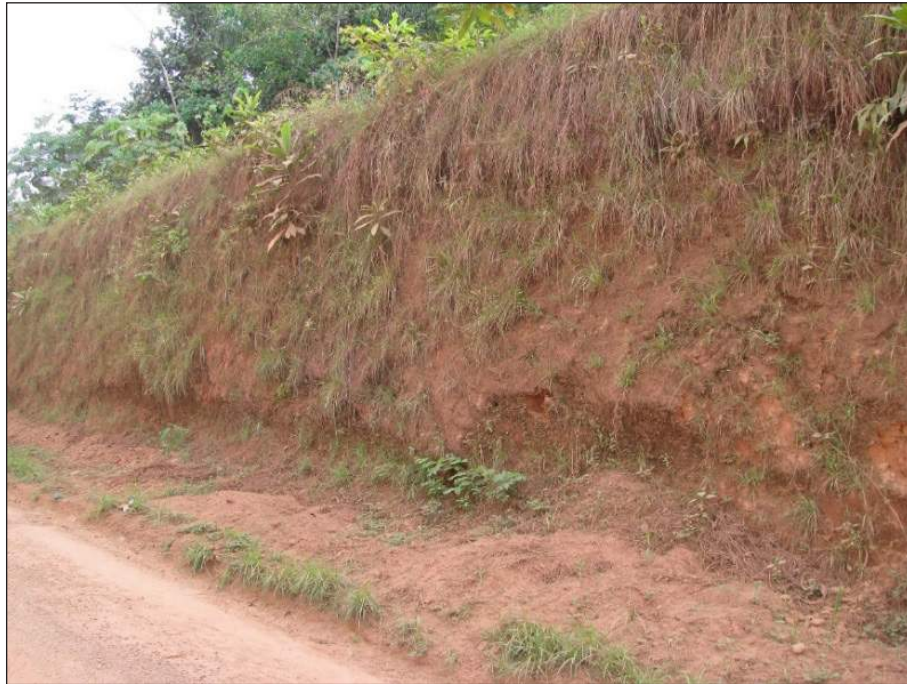
Figure C.7.7: Cut slope in WG V-VI material at 3V:1H and still intact after 40 years
