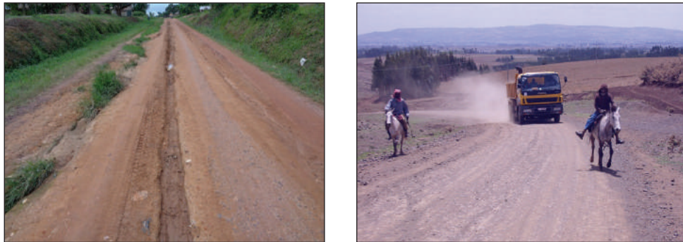
Figure E.1.4: Erosion of gravel on a hill section and dusty conditions
