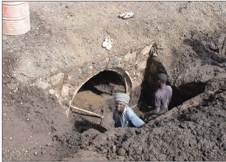
Figure E.7.2: Cleaning the drop inlet and barrel of a large bore culvert
