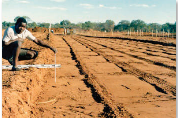
Figure B.4.12 Collapse settlement in excess of 150 mm following impact compaction
