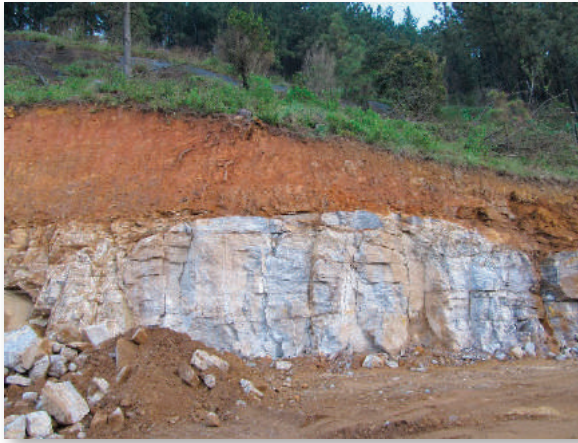
Abrupt interface between WG V and WG I-II, i.e. rock that requires blasting is found directly beneath residual soil
