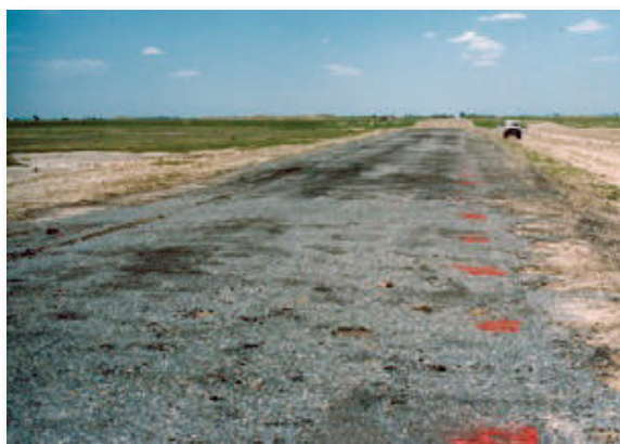
Figure B.4.15 Severe distress to a road surfacing caused by salt attack
