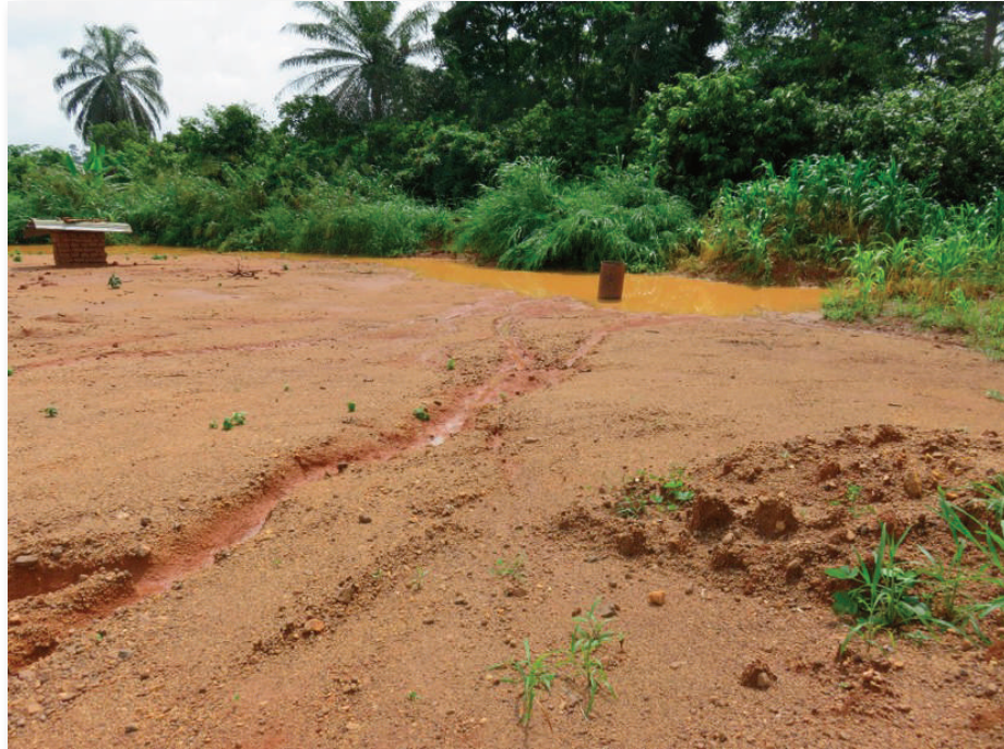
Figure B.10.3 Localised ponding in undrained low point of a borrow pit
