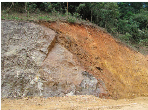
Marked lateral change from WGI on left to WG V on right with no topographic indication
