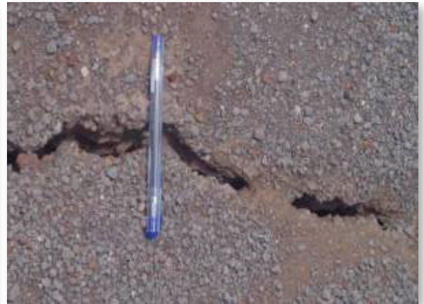
Figure B.4.7 Longitudinal cracking and deformation caused by expansive subgrade
