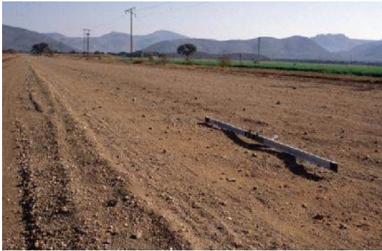
Corrugation and raveling
