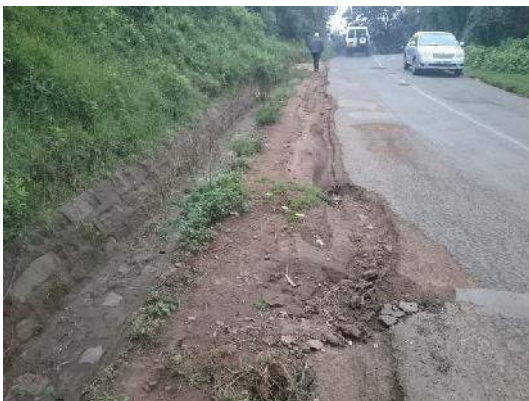
Figure 8-18: Poor – Gap between surfacing and drain lining
