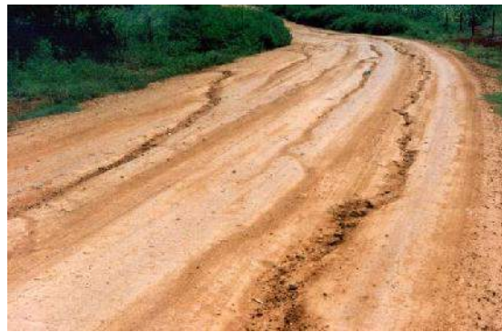
Longitudinal erosion in fine material
