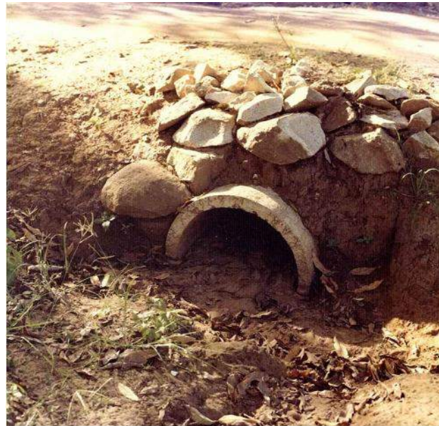
Figure 7-8: Siltation problems at culvert outlet
