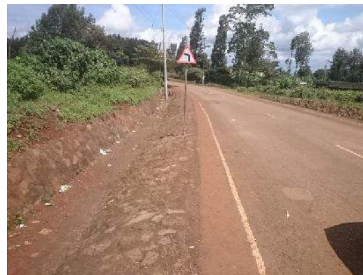
Figure 8-19: Good – Drain lining connected to edge of surfacing
