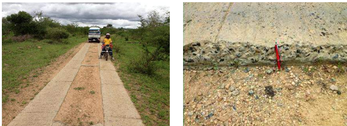
Figure 11-10: Concrete strip road with dangerous edge drop
