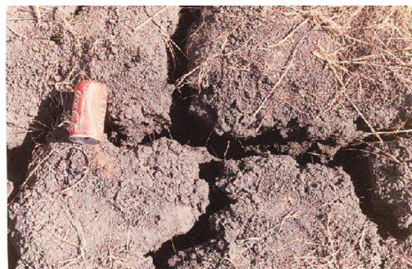
Figure 4-7: Cracking on expansive clays
