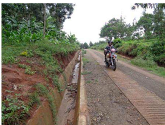
Inappropriate design of side drain
