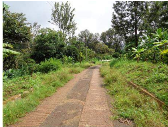
Figure 2-8: Example of poorly maintained concrete strip road
