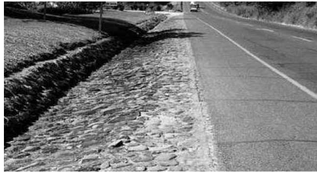
Figure 5-5: Undesirable drain design
