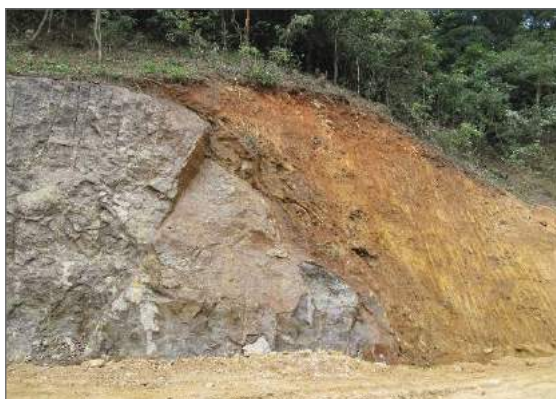
Marked lateral change from WG I on left to WG V on right with no topographic indication.
