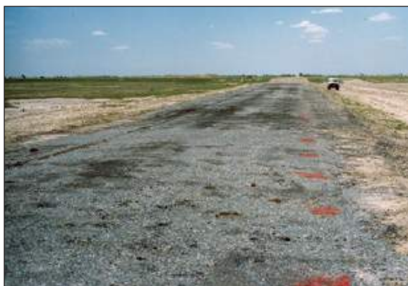
Figure B.4.15: Severe distress to a road surfacing caused by salt attack
