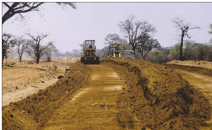
Figure B.9.10: Mixing of materials on the road with a motor grader
