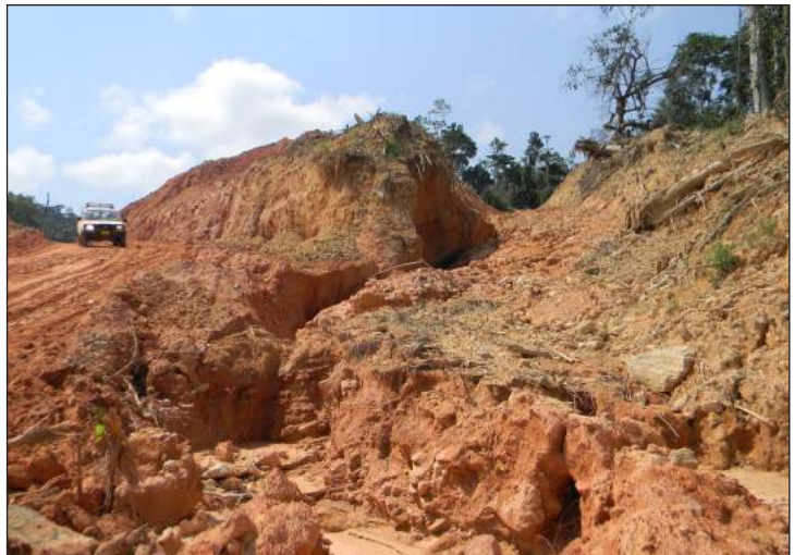
Figure B.4.14: Example of severe erosion in erodible/dispersive soils
