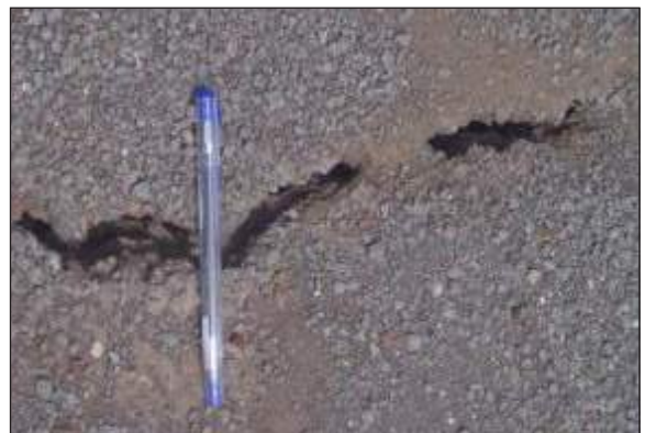
Figure B.4.7: Longitudinal cracking and deformation due to an expansive subgrade
