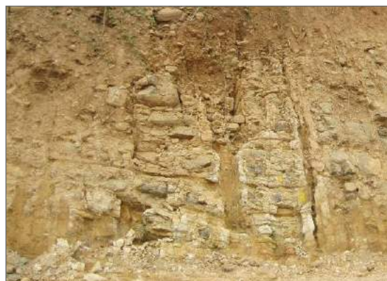
Weathering grade changes laterally as well as with depth (WG decreases in direction of arrows). Note the infilled vertical joints.
