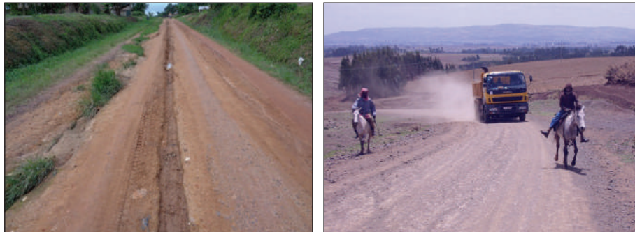
Figure E.1.4: Erosion of gravel on a hill section and dusty conditions
