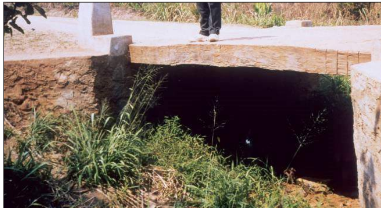
Figure E.7.1: Box culvert partially blocked by vegetation
