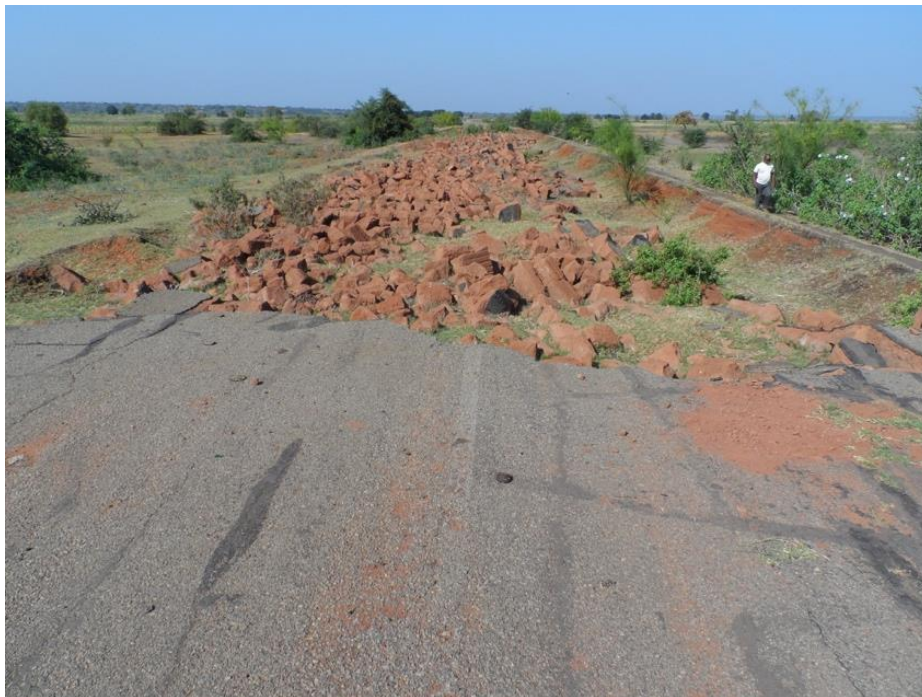
Complete loss of embankment and road due to turbulent flow conditions during overtopping and weak subbase (Courtesy Paige-Green Consulting Ltd)
