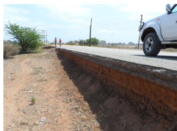
Erosion of embankment and undercutting of pavement caused by overtopping
