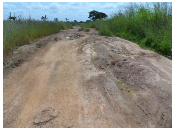
Eroded, poorly drained section of road with laterite outcrops
