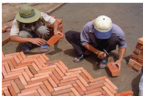
Laying bricks in 'herringbone' pattern between previously laid kerb edge restraints (bricks bedded and jointed in sand-cement mortar, on a conventional road base).
