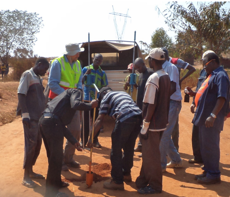
AFCAP consultants and local partners collect data using Dynamic Cone Penetrometers and augers on the Kalemie-Uvira road in Katanga Province.
