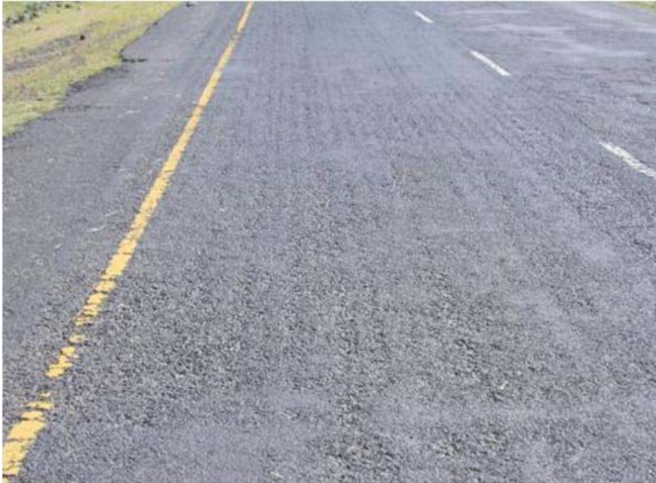
Aggregate stripping due to poor binder transverse distribution
