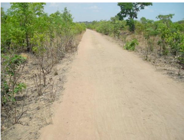
Plate 5 – RD592/2 – due for maintenance – narrow carriageway
