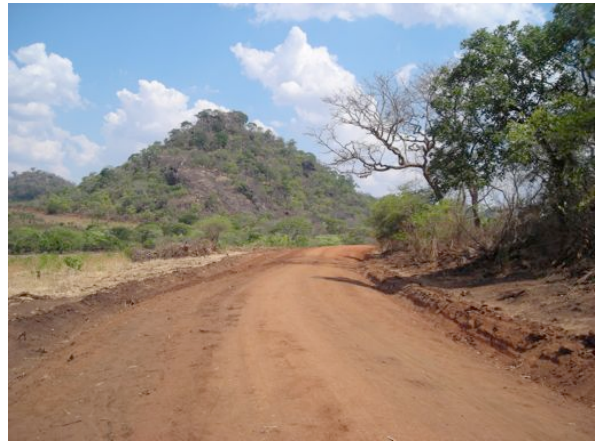
Plate 8 – RD687 – section due for maintenance, some of which is in very poor condition
