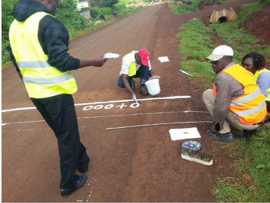
Figure 13: The solid line with chainage 0 + 000 marking the beginning of the section to be monitored
