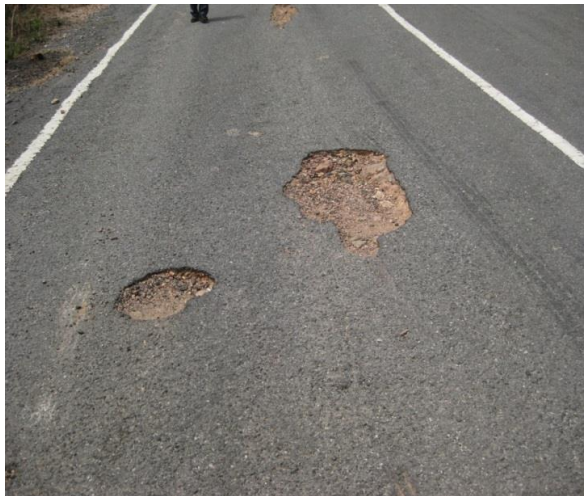
Potholes on Bituminous Surface Due to Traffic Action - Aprade-Somanya Road Section
