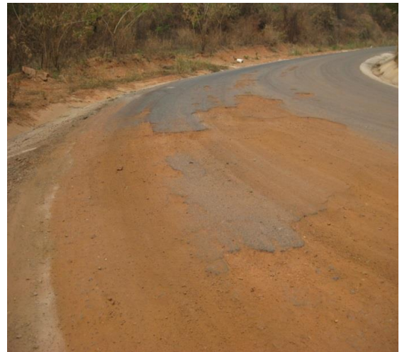
Surface Failure of Single Seal Section on the Somanya - Oterpolu Road
