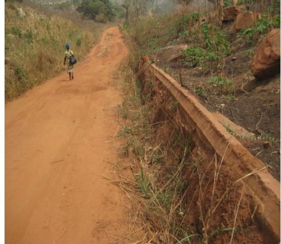
Severe Erosion Renders Kerbs Non-Functional: Teiwanya-Sekasua Road Section
