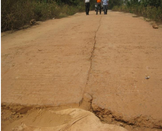
Partially failed concrete structure showing longitudinal and transverse cracks
