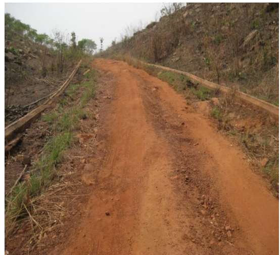
Run-offs from cut sides caused serious road surface erosions - Teiwanya – Sekasua
