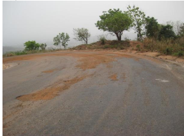
Eroded Single Seal on Sharp Curve, on Steep Slopes: Somanya-Oterpolu Road Section
