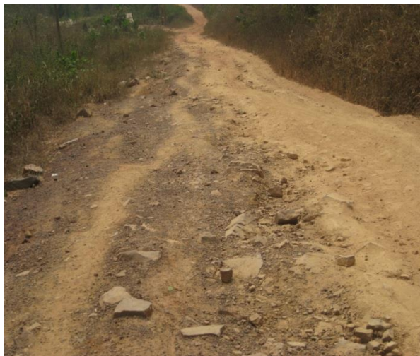
Exposed stones (100mm) due to erosion on the Klo Agogo – Oluhai section
