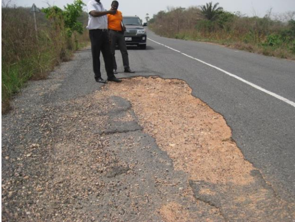
Spalling of Single Seal Surfacing on: Aprade-Somanya Road Section
