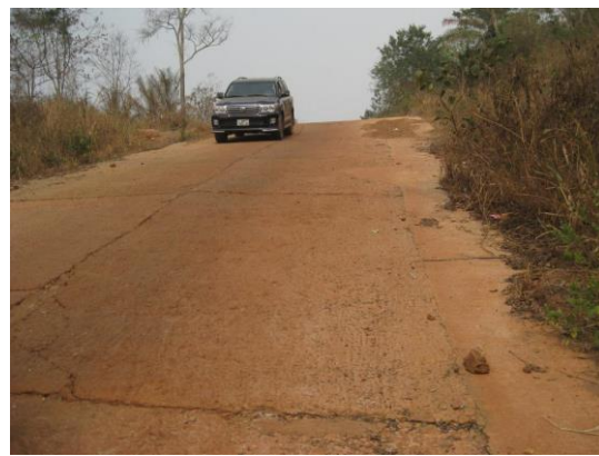
Sever Block and Corner Cracks Road Section
