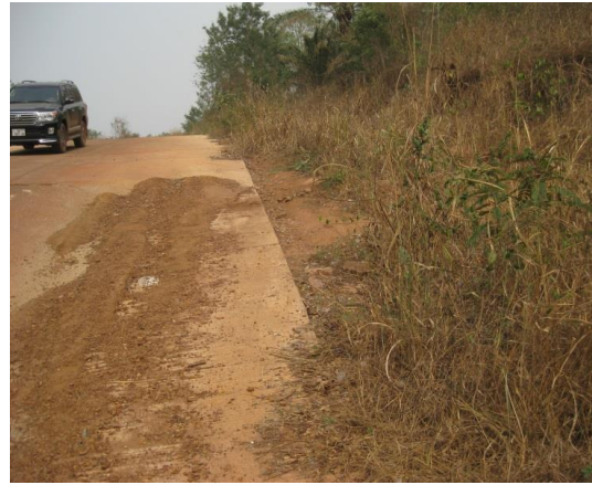
Washed material from cut surface on the road: Tafo – Nobi road section
