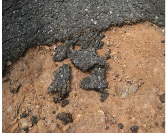
Disintegration of Single Seal Surfacing on Somanya - Oterpolu Road
