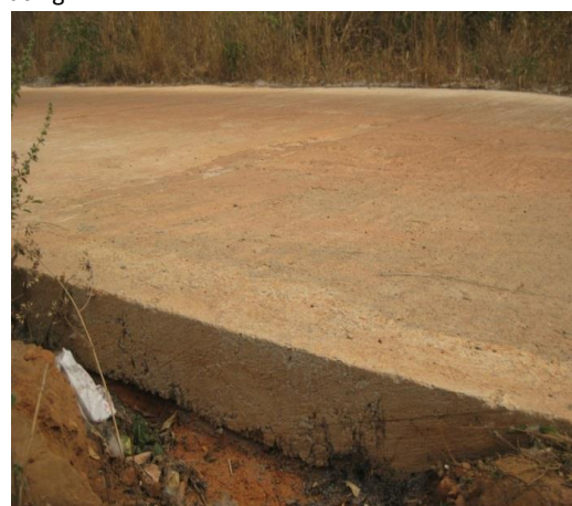
A 200 mm Thick Reinforced Concrete on a Steep Section of Agogo-Opesika Road
