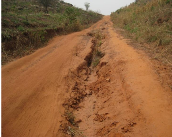
Erosion Caused Gullies On Teiwanya-Sekasua Road Section
