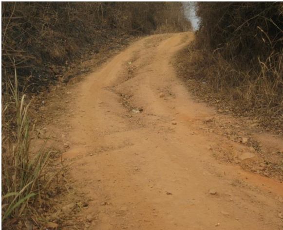
Erosion, Gravel Loss on Teiwanya-Sekesua Road Section
