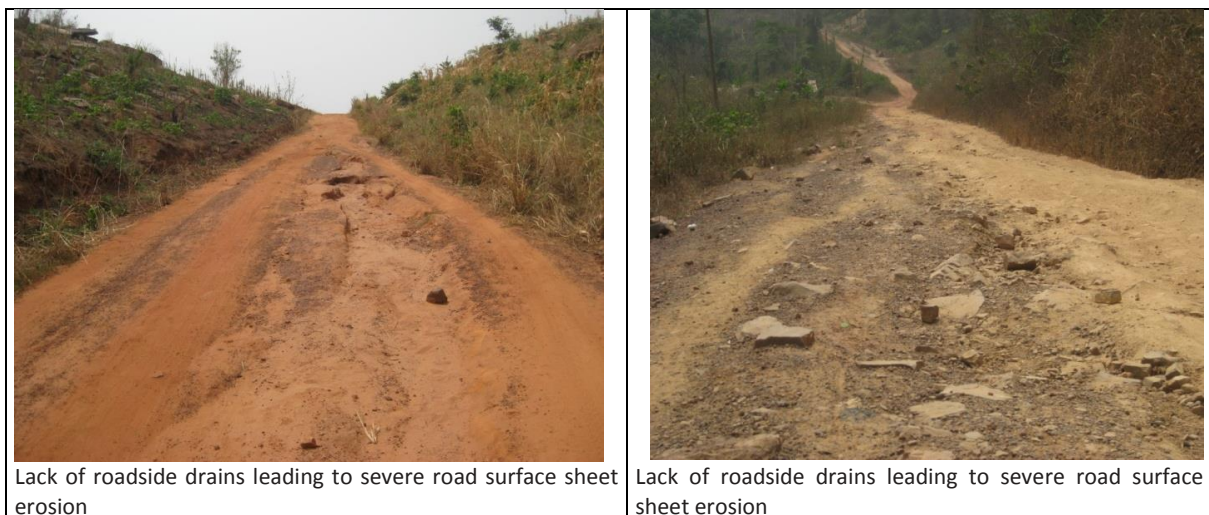
Figure 6-1: Severe road surface (sheet) erosion on gravel roads
