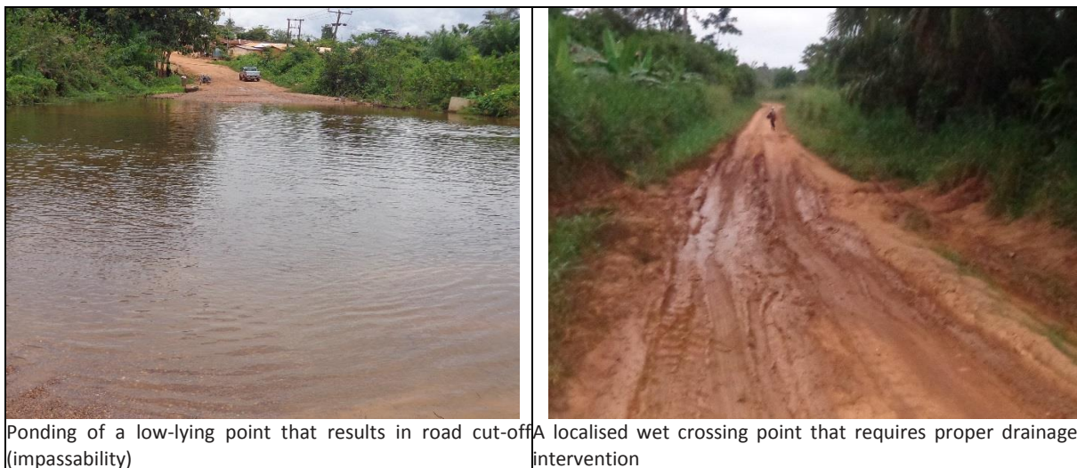
Figure 6-4: Drainage problems at the trough (base) of slope sections
