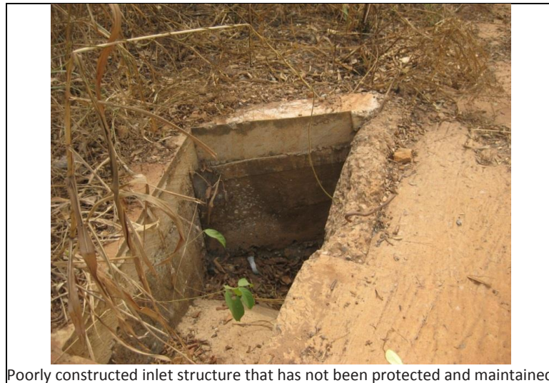
Figure 6-5: Drainage problems at the trough (base) of slope sections
