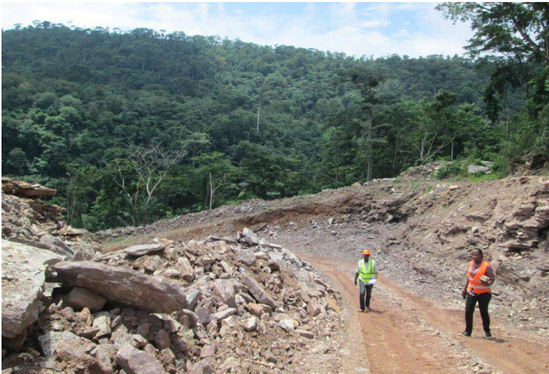
Figure 22: Road section on a slope ~18%, and a curve, requires safety considerations
