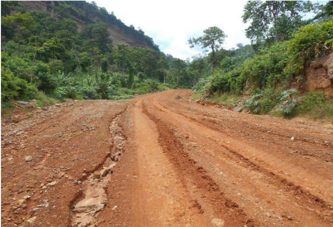
Figure 23: Early erosion signs of road surface due to steep slopes on gravel surface
