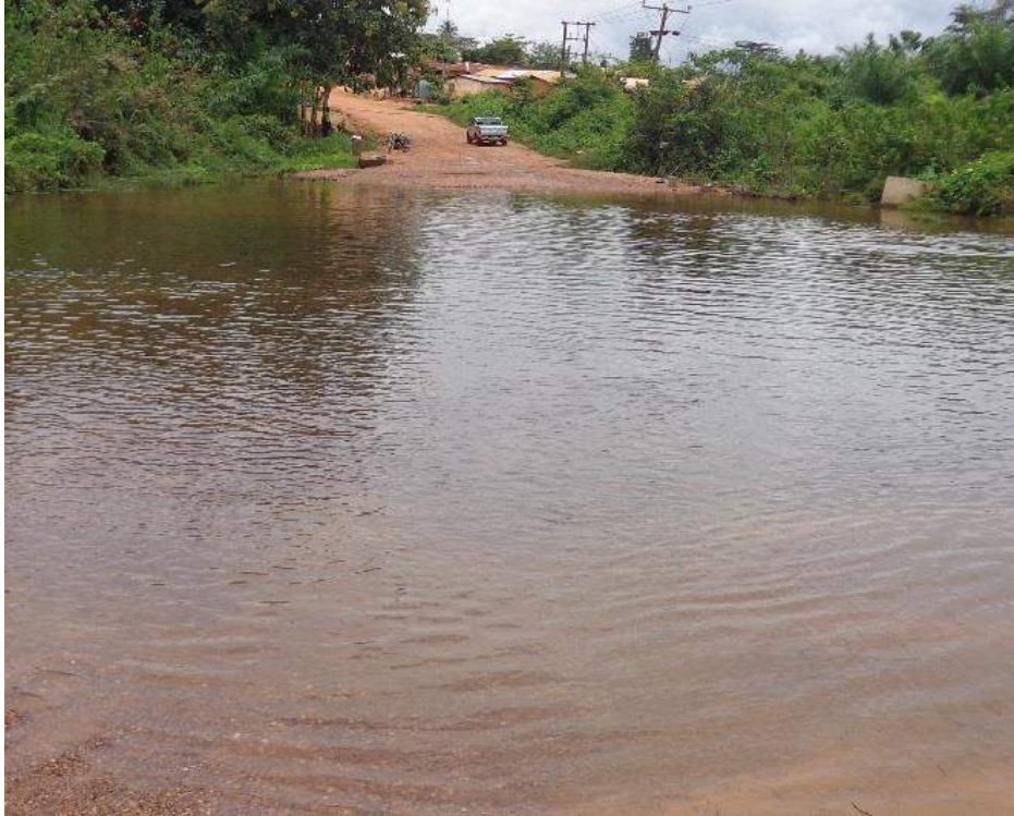
Figure 2: Flooding on a feeder road—requires intervention
