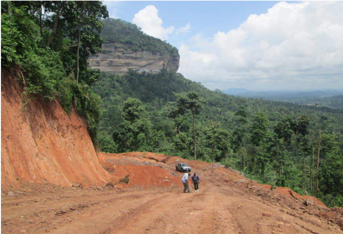
Figure 21: Road section on a slope ~16%, and a curve, requires safety considerations
