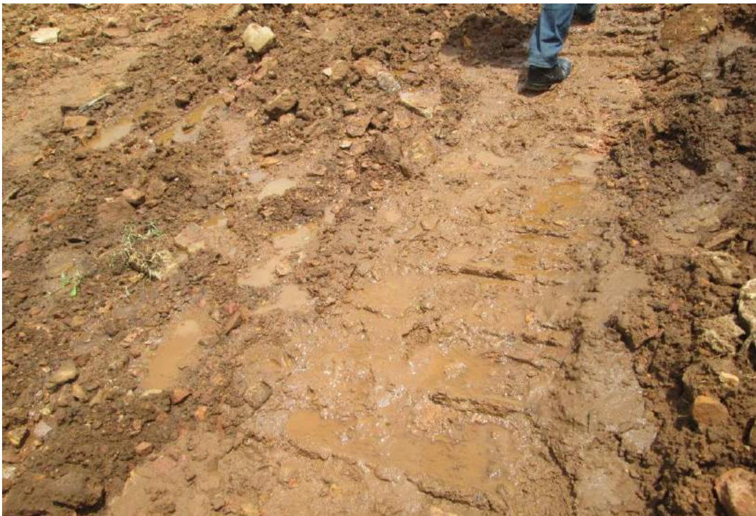
Figure 24: Prepared road foundation damped due to ground water action
