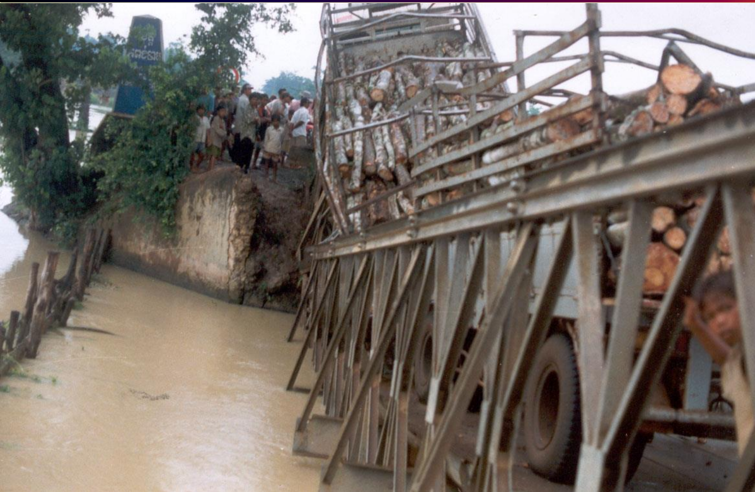
Collapsed Bridges on RN6 and RN7
