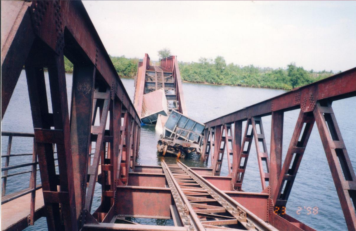
Collapsed Bridge on Rail Bridge
