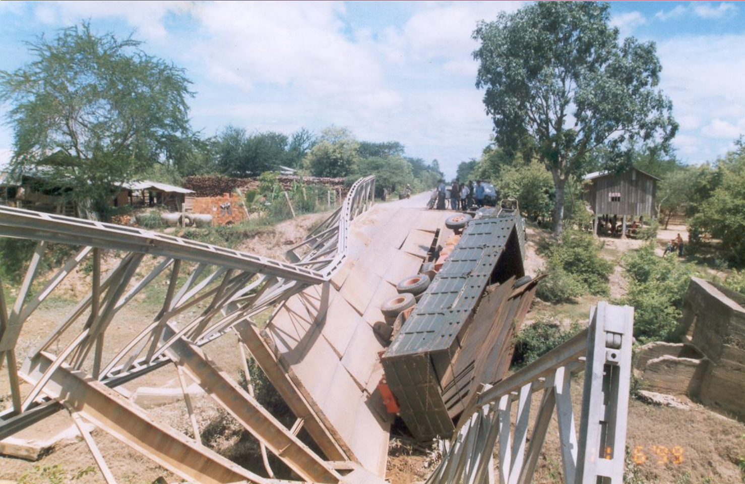
Collapsed Bridges on RN3
