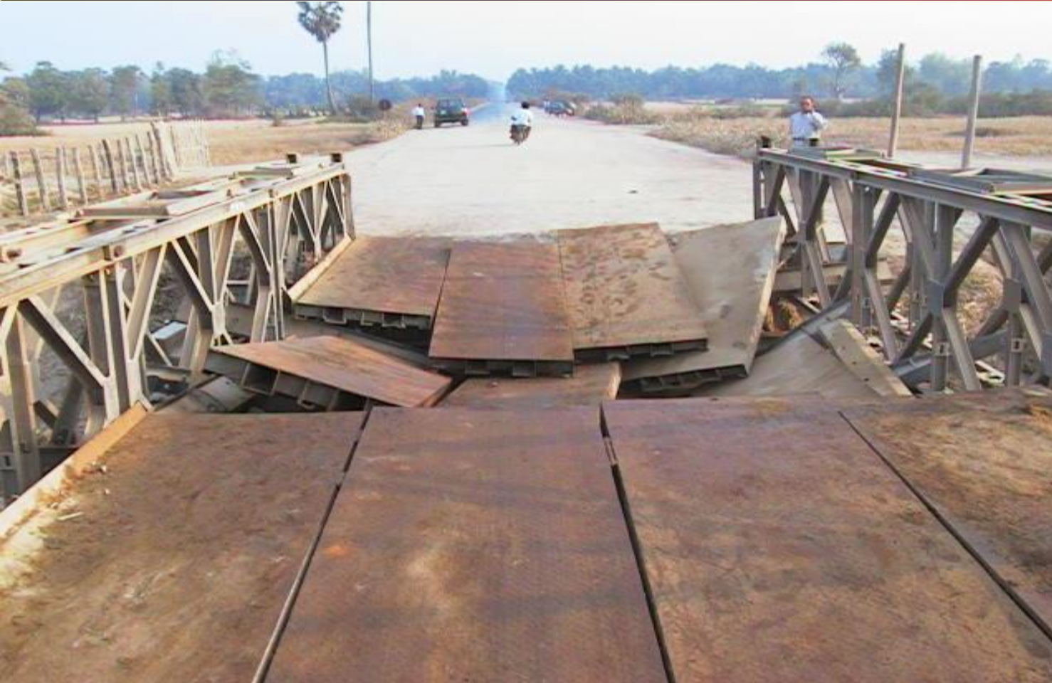
Collapsed Bridges on RN5
