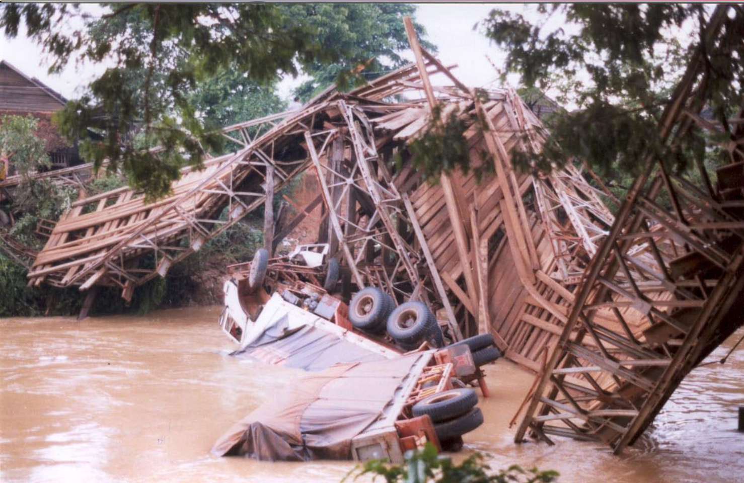
Collapsed Bridges on RN6 and RN7
