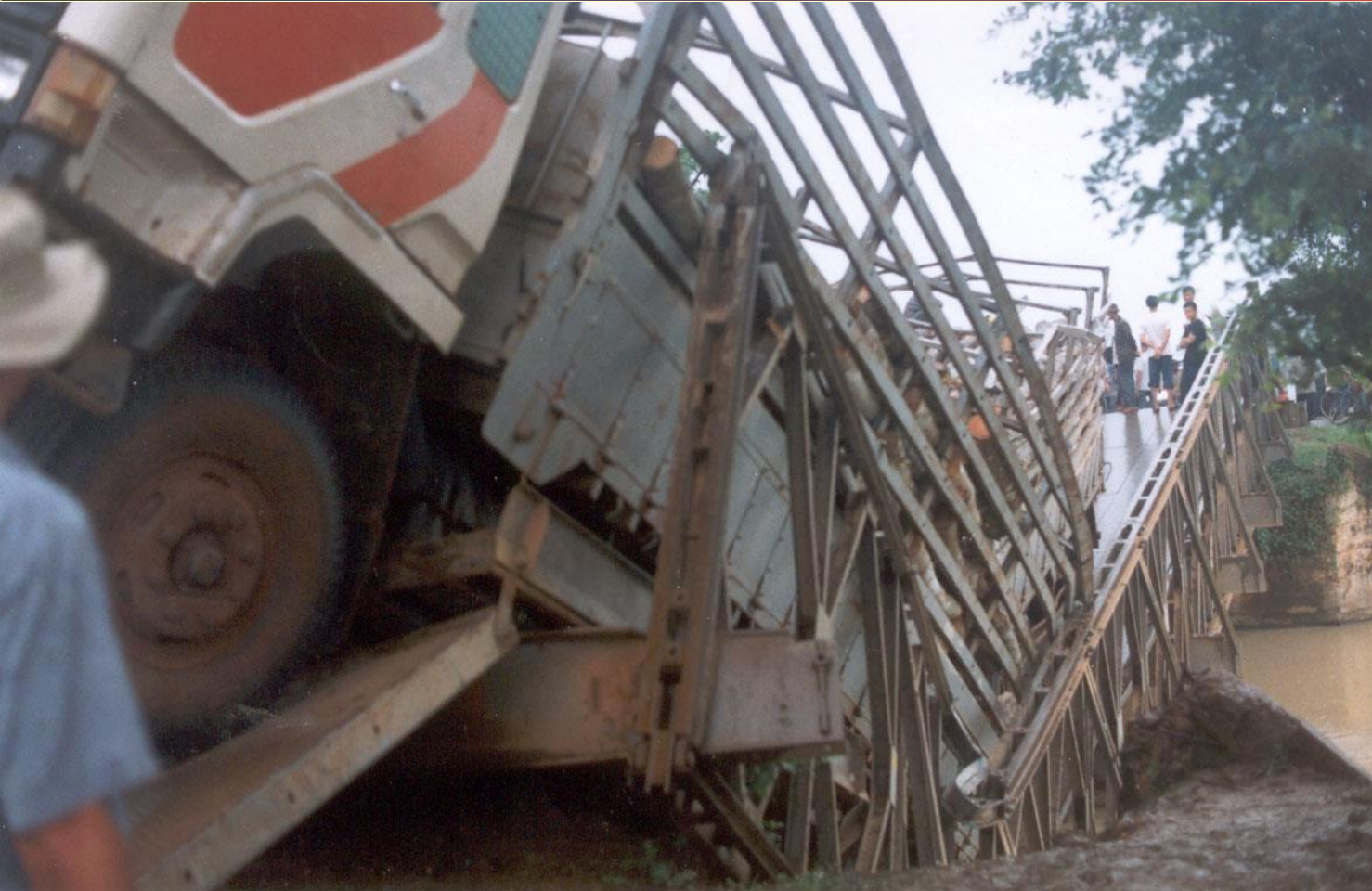
Collapsed Bridges on RN6 and RN7
