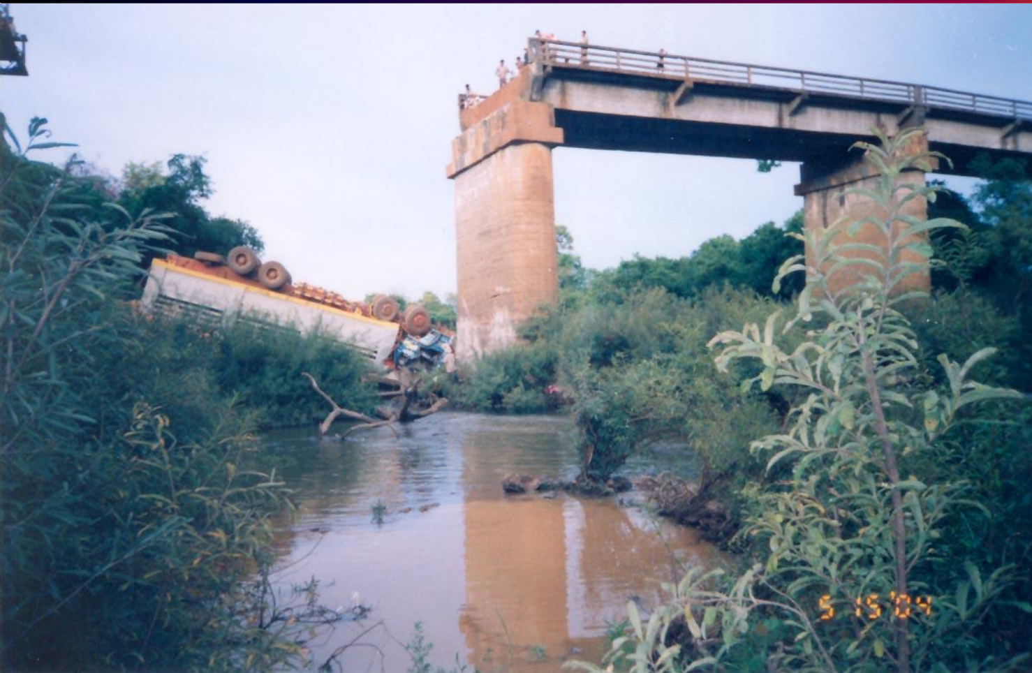
Collapsed Bridges on RN6 and RN7
