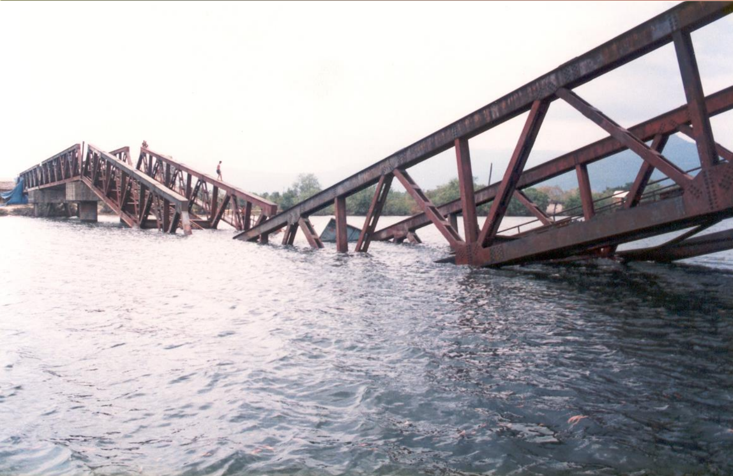
Collapsed Bridge on Rail Bridge
