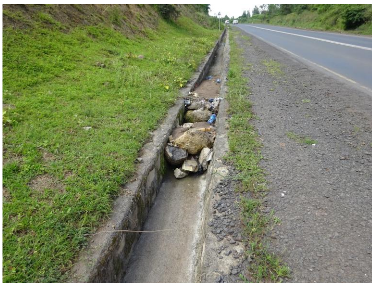
Figure 15 Unpaved area between impervious seal and lined drain allowing access of water into the pavement (Note poor maintenance of side drain as well)
