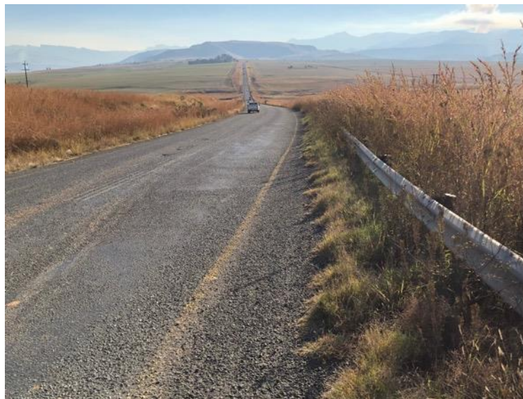
Figure 28 Thick vegetation alongside road indicating insufficient maintenance (rated at 5/5)
