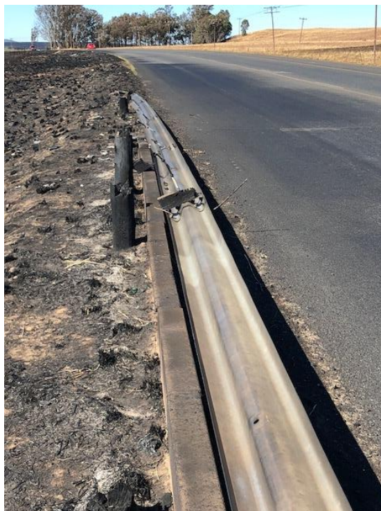
Figure 30 Damage to guardrail posts and bitumen surfacing caused by wildfire
