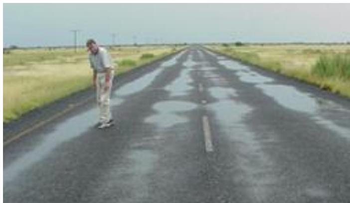
Figure 8 Typical manifestation of collapsible soils in paved road
