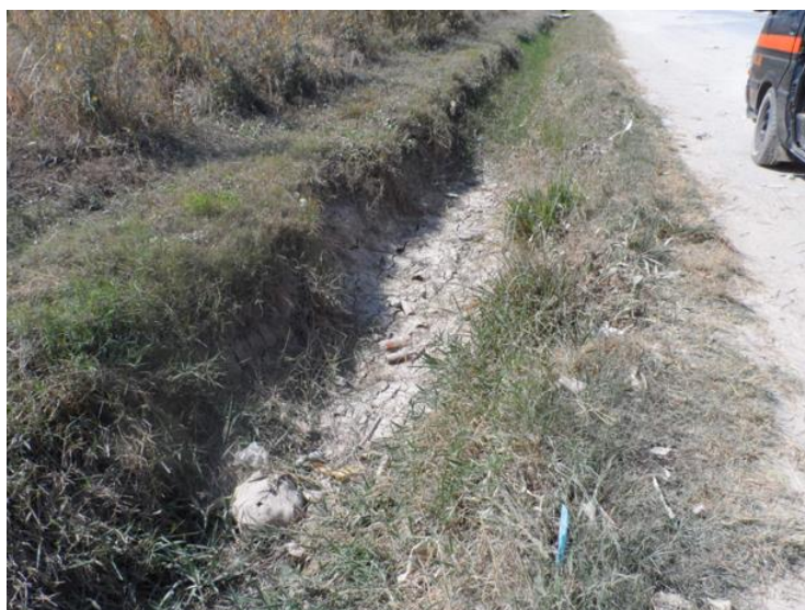
Figure 11 Evidence of ponding of water in side drain
