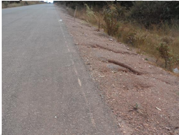
Figure 26 Poor finish of newly constructed road
