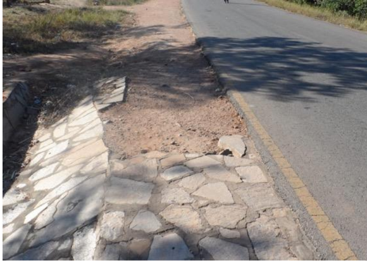
Figure 27 Poor finish of protection works resulting in failure – no “anchor” beams
