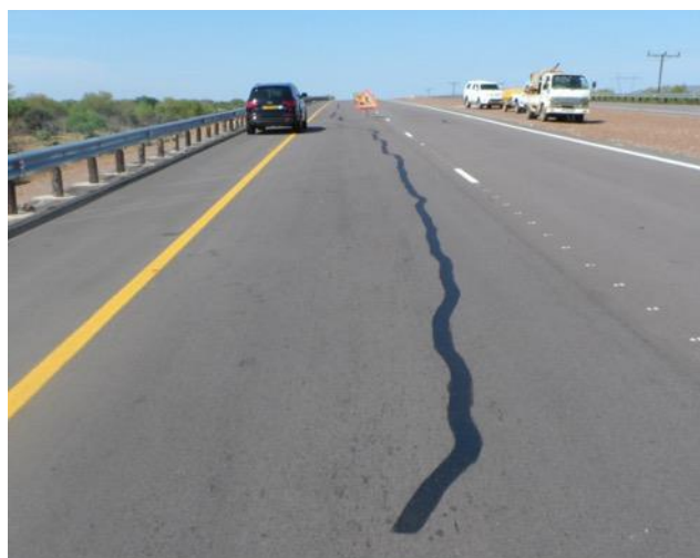
Figure 24 Cracking of embankment due to overstressing
