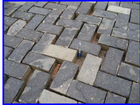
Plate 4: Seal Eroded from Concrete Block Paving: Sand Joints
