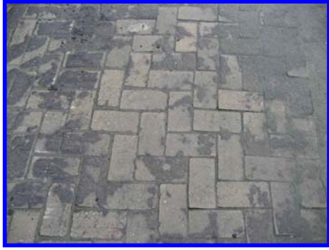
Plate 3: Seal Eroded from Concrete Block Paving: Mortar Joints
