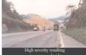
High severity resulting in severe ride
