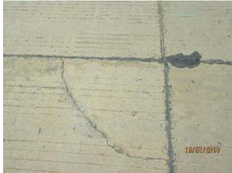
Corner crack in concrete slab
