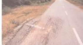
Moderate severity resulting in rough ride
