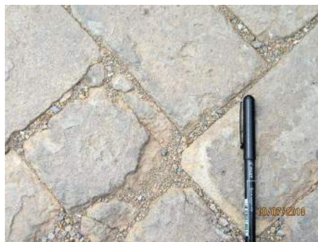
Concrete Block Breakage
