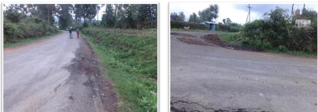
Figure 7: Failures induced by heavy vehicles at the junction with main road
