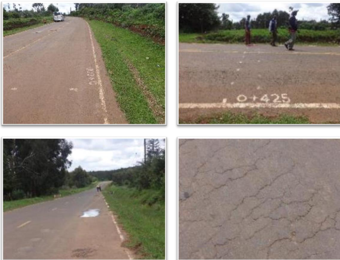
Figure 3: Road condition D382
