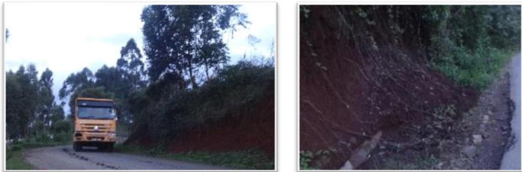
Figure 6 : Construction traffic on Kangari-Kinyona Road and Slope Failure
