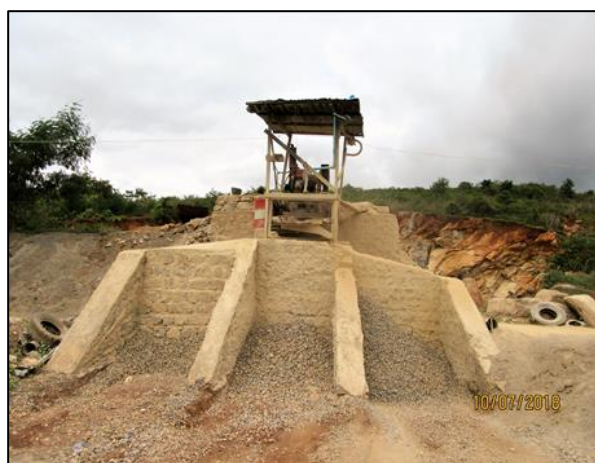
Single stage crusher adjacent to the site
