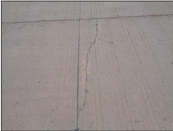
Crack in concrete slab
