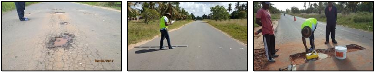
LTPP Section 2 deteriorating rather quickly
