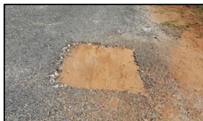
Test pits excavated in February yet to be properly backfilled and sealed
