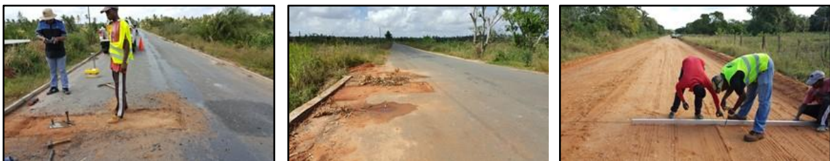
Preparation for measurement of insitu moisture content and density on LTPP sect. 2
