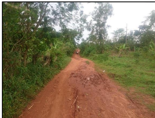
Figure 4: Poor Drainage on Nawatale – Kibuye Road, Kamuli District
