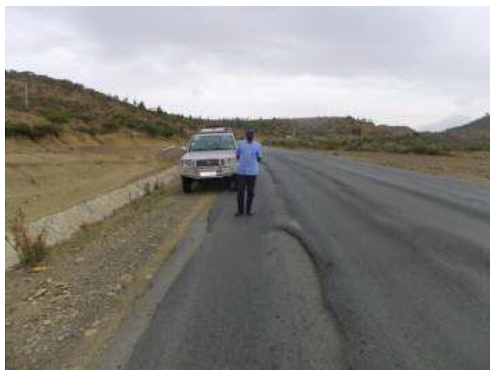
Figure 7-1 Deformation of the AC surfacing on the Mekelle - Combolcha road
