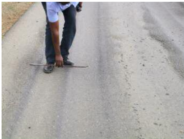
Figure 7-2 Rutting in the wheel path on the Mekelle-Combolcha road
