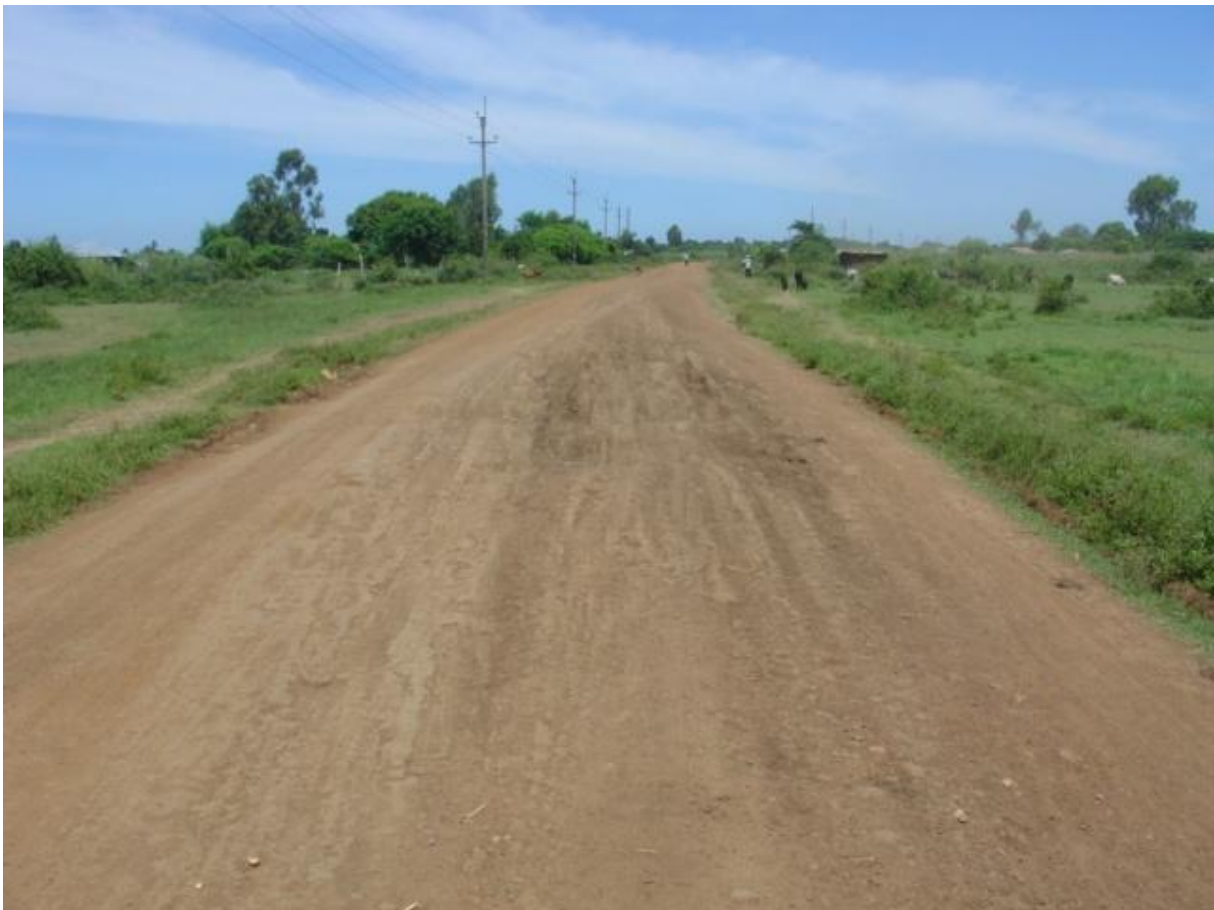
Picture 1: Typical flat section on the Nyenye branch with damage in the black cotton sub-grade from the rainy season
