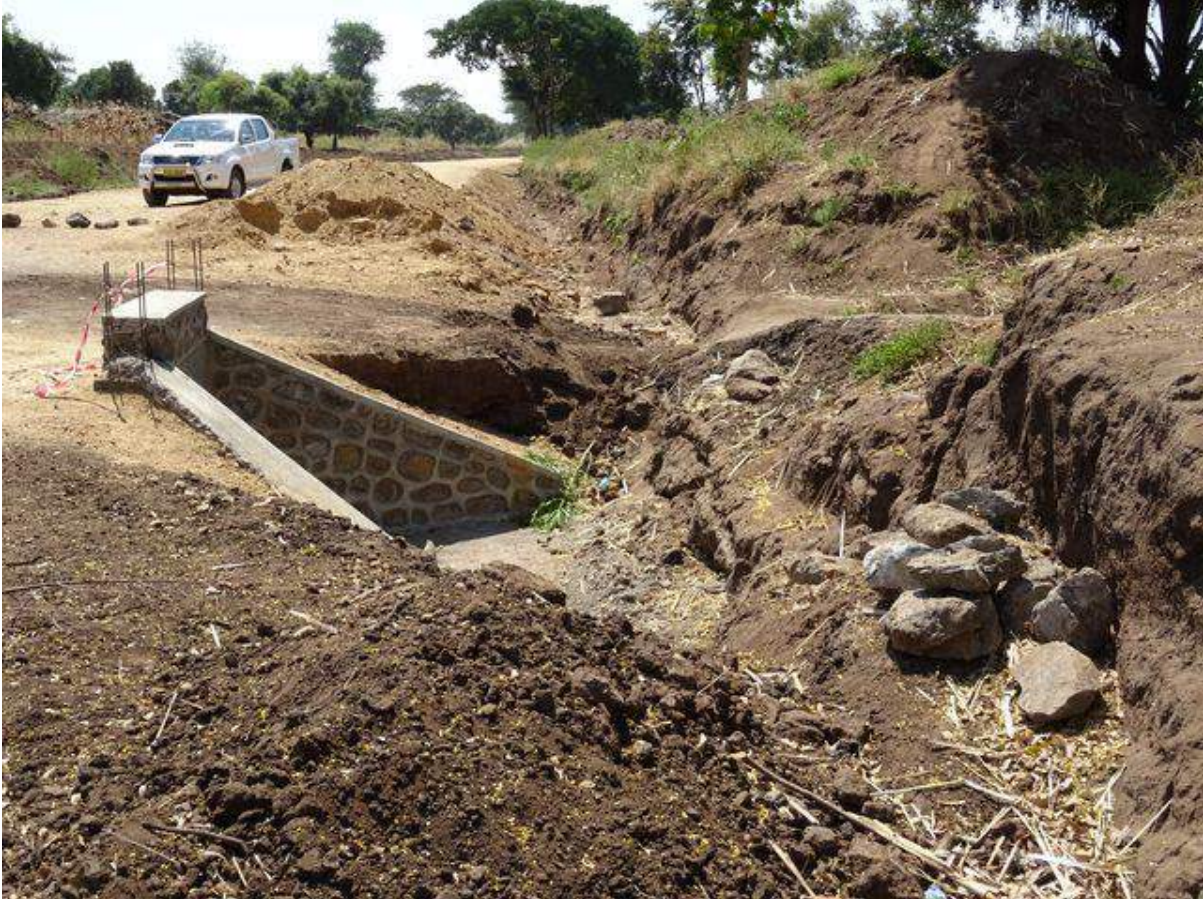
Figure 4: S134 Kasinje – Kandeu. New culvert with invert well below side drain invert. Road level well below surrounding ground.
