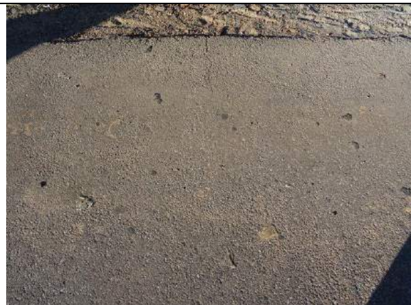
Figure 10: Small defects in CMA
