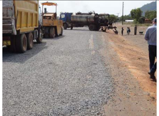
Figure 7: Patch not covered with bitumen, loss of aggregates
