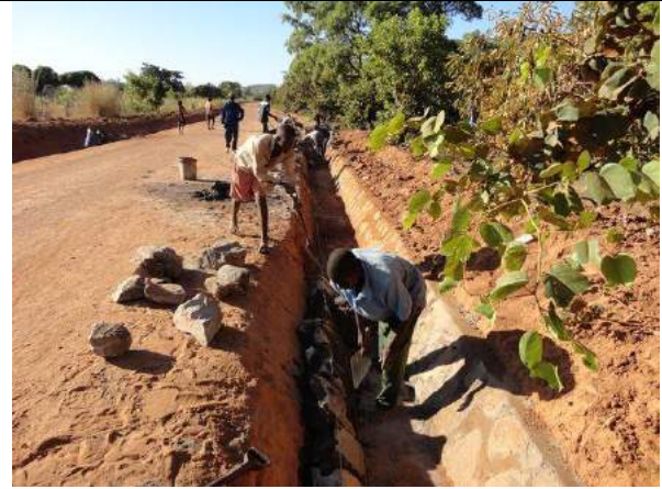
Figure 15: Narrow drain with steep sides
