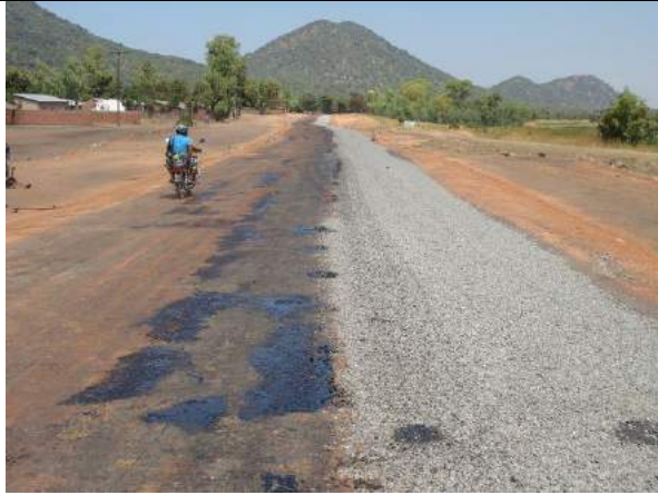
Figure 6: Patchy work and irregular lines
