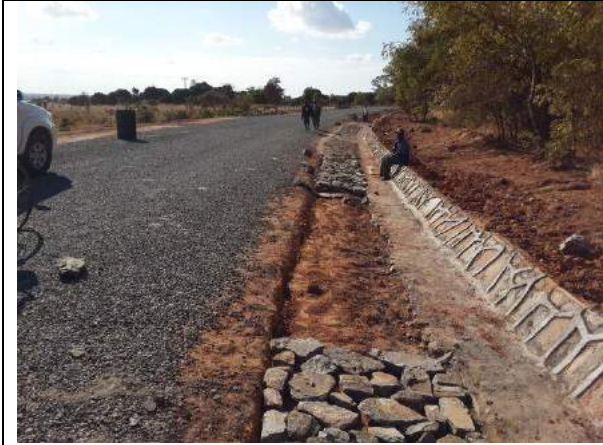
Figure 14: Gap between drain lining and surfacing. Wide, shallow drain
