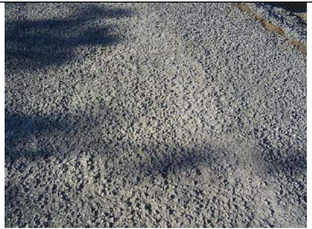
Figure 9: Uneven surface due to irregular bitumen spray rate
