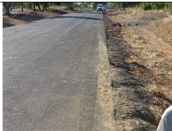
Figure 12: Wheel track on loose shoulder
