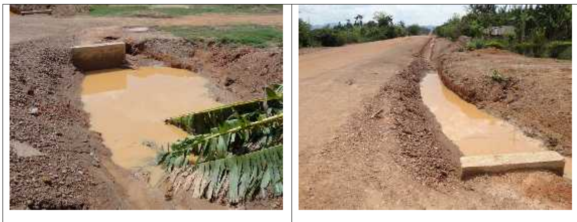
Figure 14: Access culvert at km 8+700 LHS must be replaced with new culvert or dish drain at correct invert level
