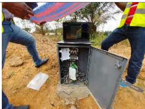
Figure 24: Data loggers connected to all sensors
