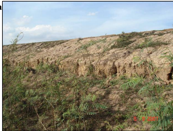
Figure 3. Illustration of Wave Erosion on a Section of RN 8 in Prey Veng.
