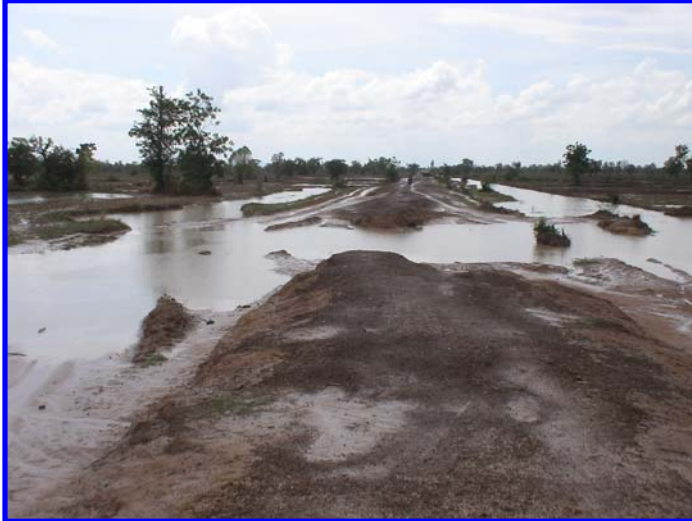
Photo 1 Eroded Gravel Road
