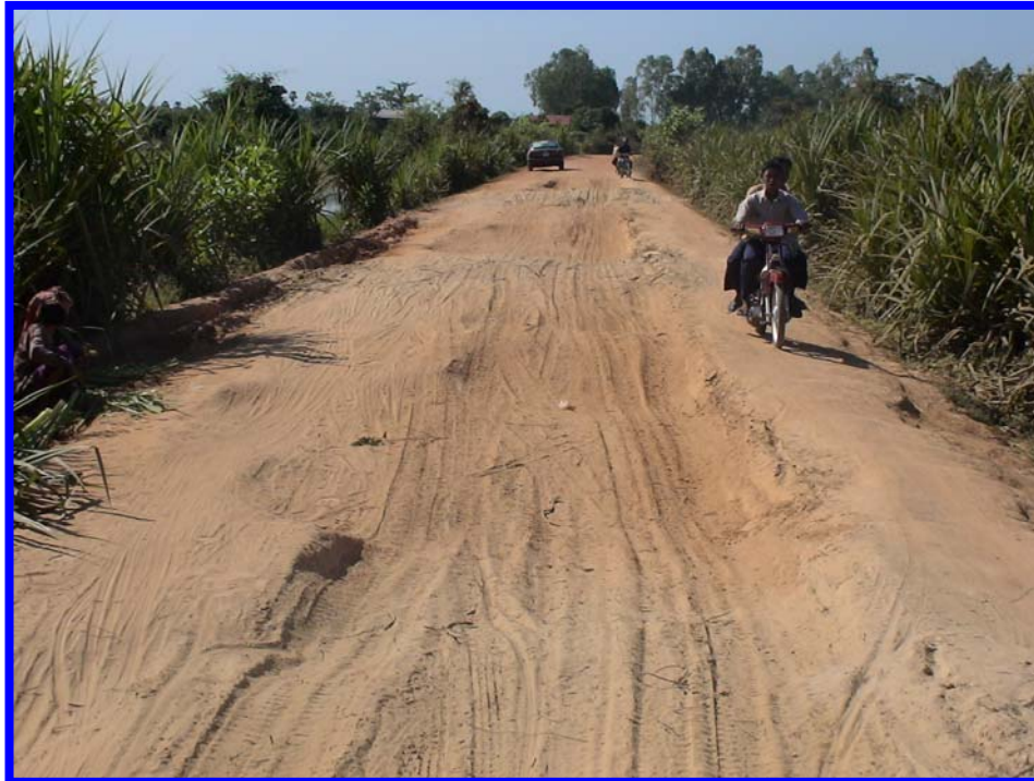
Figure 2.3 – A donor funded project gravel road within 2 years of maintenance cessation (dry season and impassable by motor car!)
