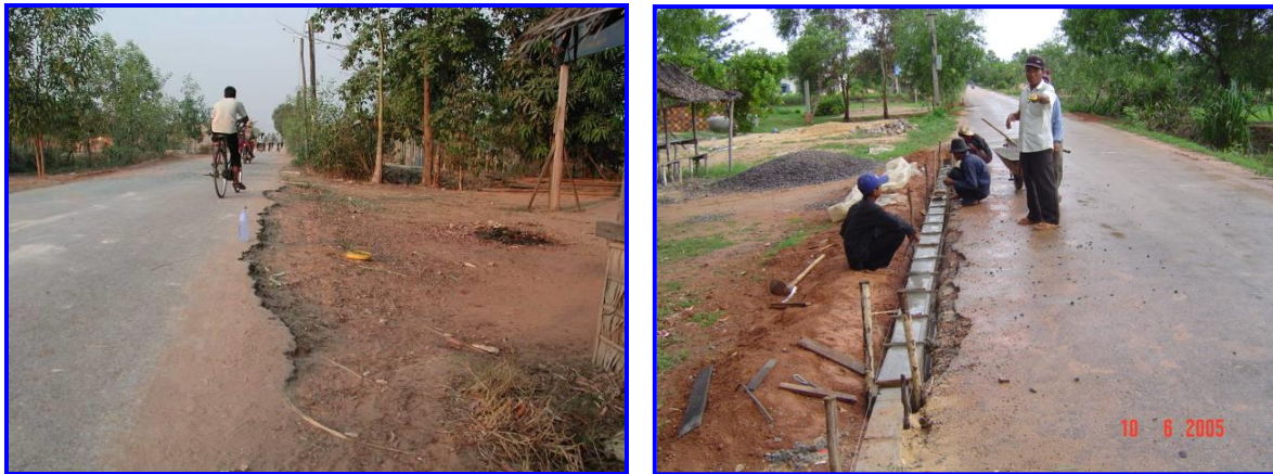
Figure 5.3 & 5.4: Edge failure and construction of flush concrete kerbs
