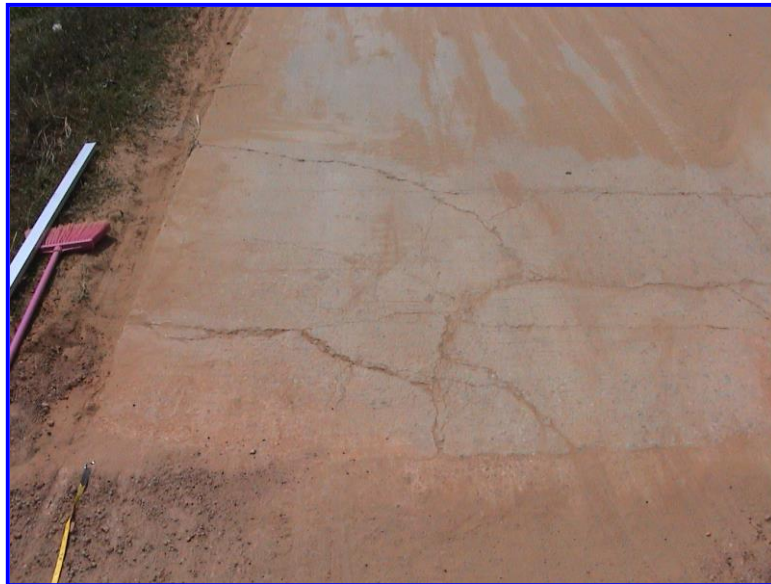
Figure 6.1: Final BRCP slab of ILO paving trial which had suffered cracking due to high impact loading by heavy trucks.
