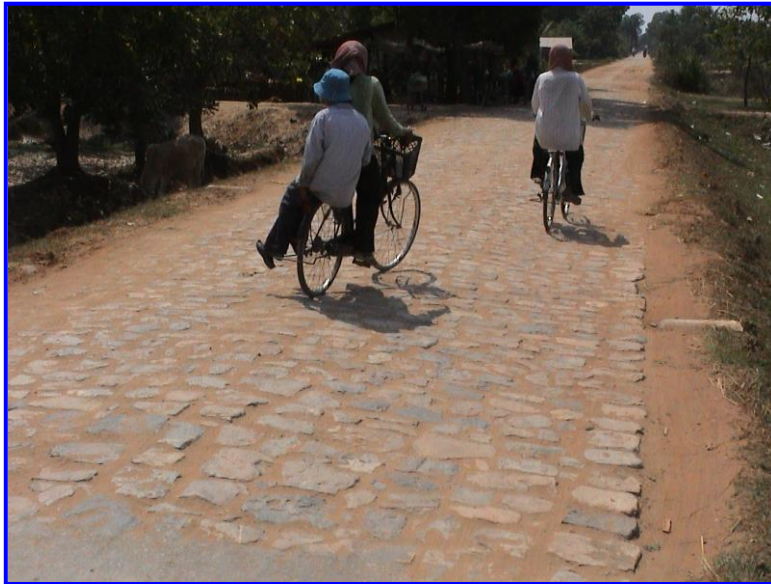
Figure 6.2: Dressed Stone Paving Section 5 before Phase II overlay work (note the previously installed concrete obstructions to deter shoulder use)
