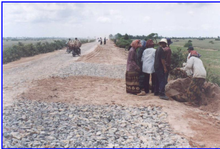
Figure 5.1: Poor Macadam roadbase construction technique filling the voids between stones with plastic fines
