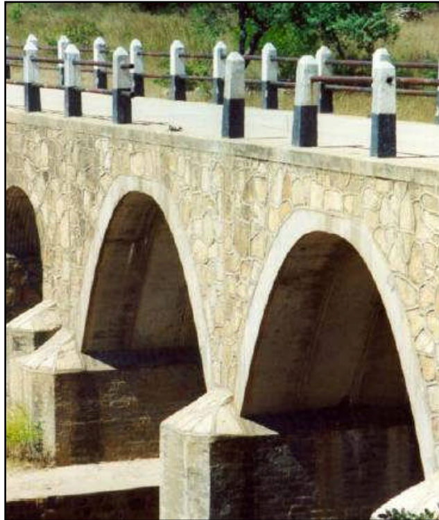
Figure 3.6 Pedestrian guard rails (in need of repair)
