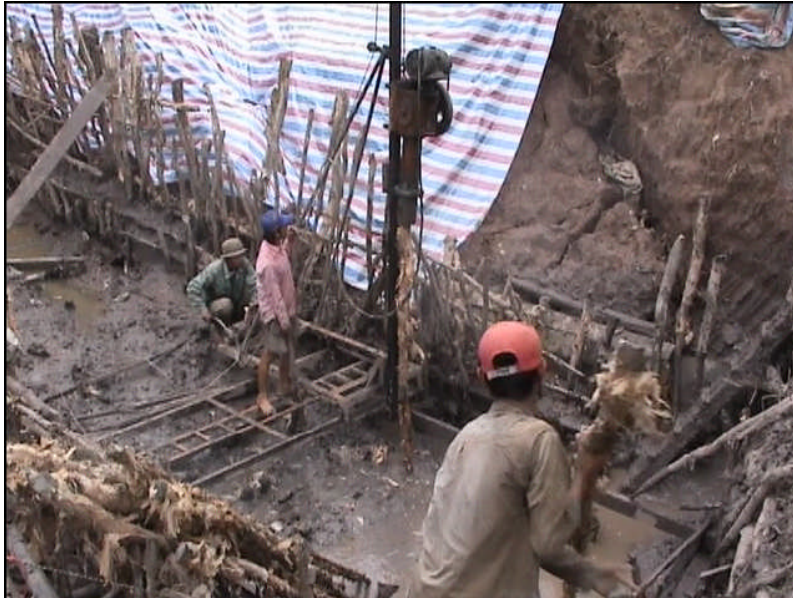
Figure 5.5 Timber piles being driven into very soft ground for a culvert foundation (requires specialist expertise, not covered by this guideline)
