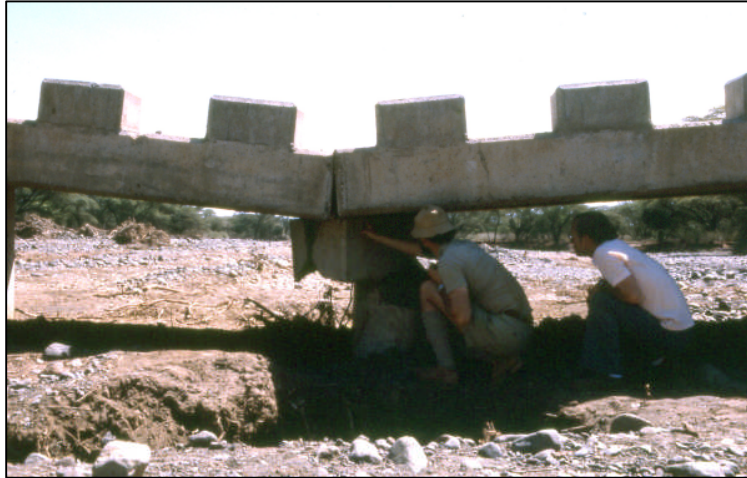
Figure 5.4 Collapse due to settlement
