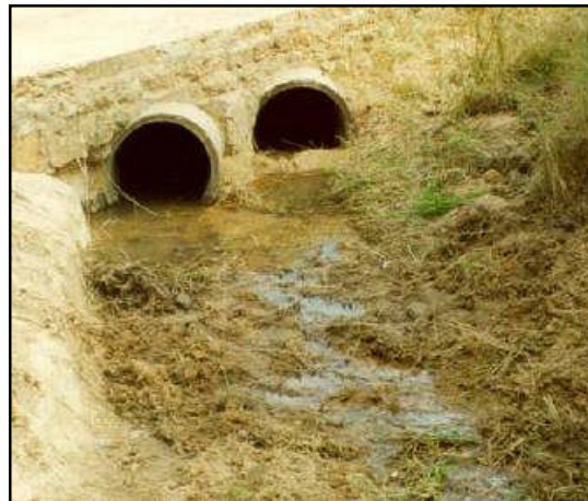
Figure 5.7 Ponding at culvert outlet
