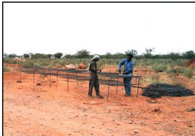
Figure 7.47 Steel reinforcement cage being assembled for the cut-off wall in a drift
