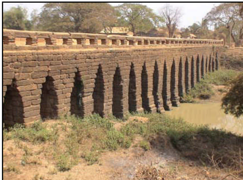
Figure 7.2 Dry jointed, laterite, stone viaduct, approximately 1,000 years old, still in service on a national main road.
