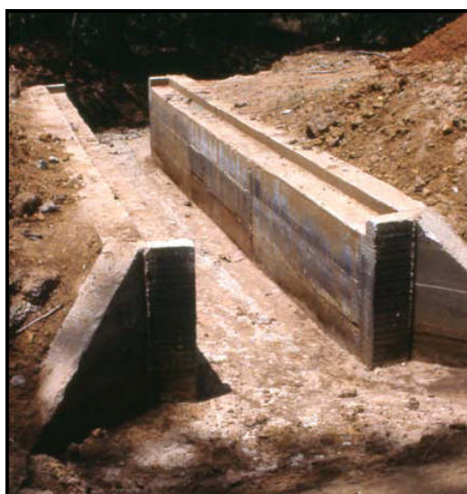
Figure 7.54 A simple reinforced concrete walled box culvert ready to receive pre-cast top slab units (timber or reinforced concrete).
