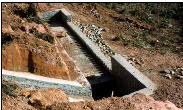
Figure 7.53 Flow spreader structure at the outlet of a mitre drain on a steep fragile slope. Bio-engineering planting should be established downhill of such structures.
