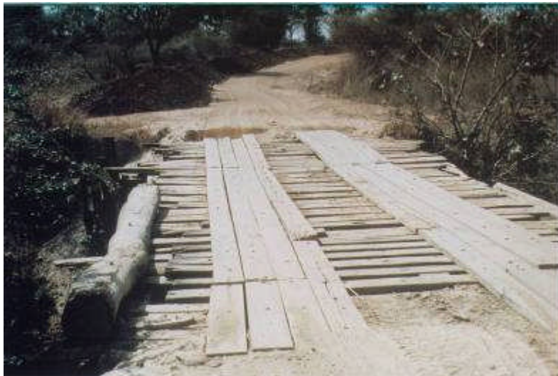
Figure 8.57 Timber deck with floor planking and edge beams in need of repair
