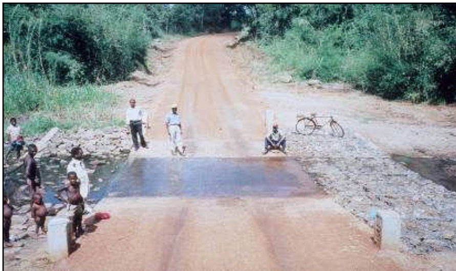
Figure 8.6 Concrete slab drift
