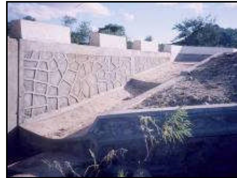
Figure 8.38 Masonry side drains at the edge of an approach way to prevent erosion
