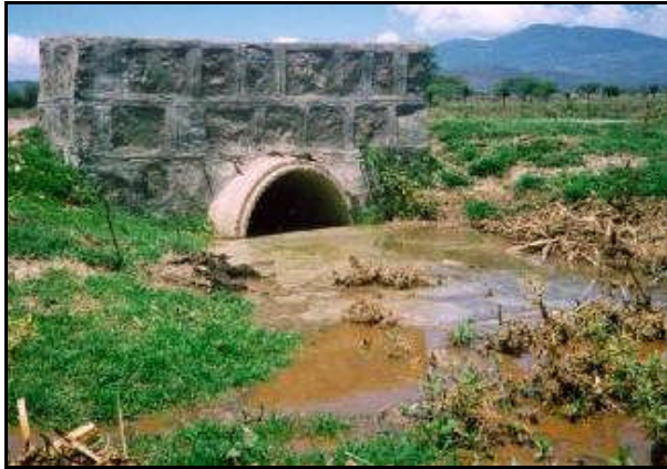
Figure 8.13 Ponding at culvert outfall
