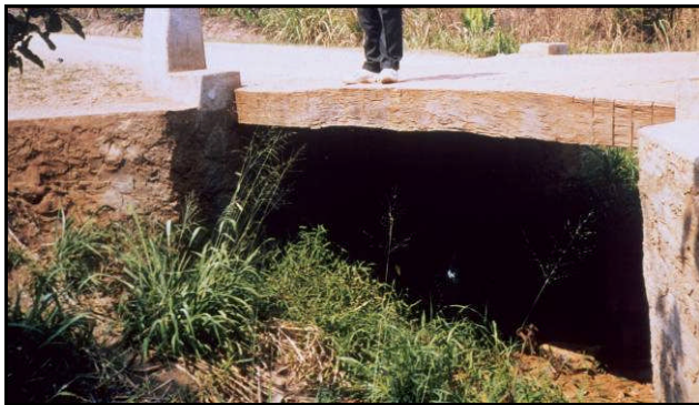
Figure 10.3 Box culvert partially blocked by vegetation
