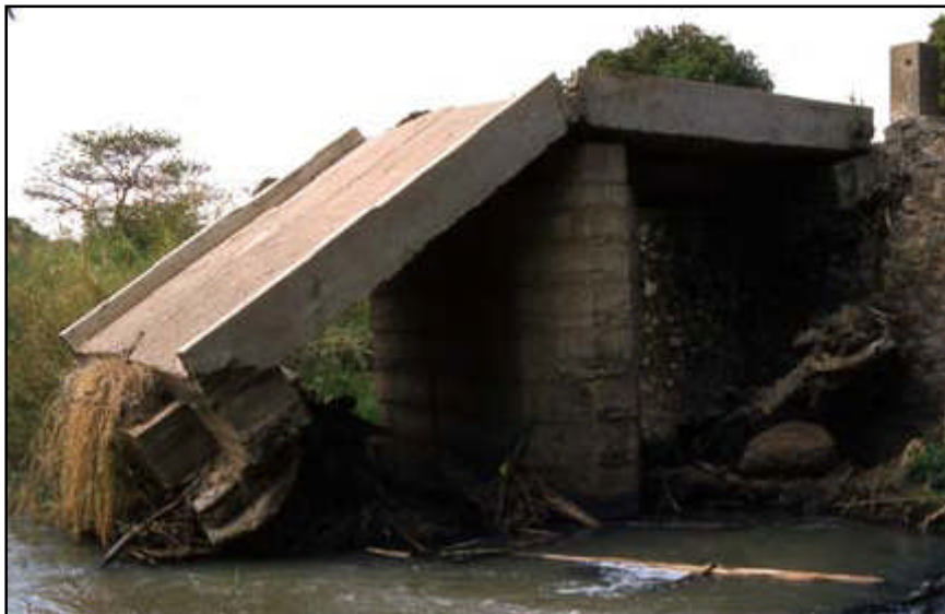
Figure 8.3 Failure of structure due to a combination of constriction of the watercourse (structure too small), scour and inadequate protection of abutments.
