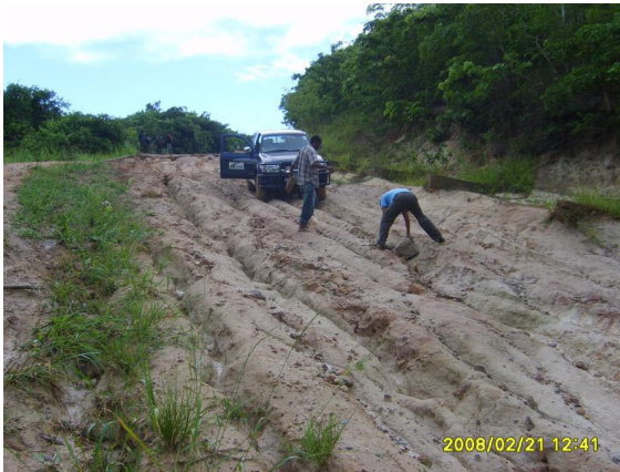
Photos n° 13: Before intervention, Feb 2008
