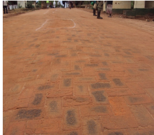
Photo nº 2: Visual signs of bricks wearing off
