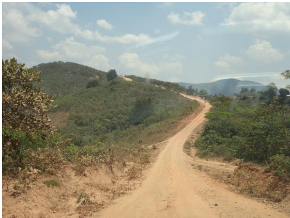
Picture 3: Typical section of D11 with steep grades up to 20% in short sections
