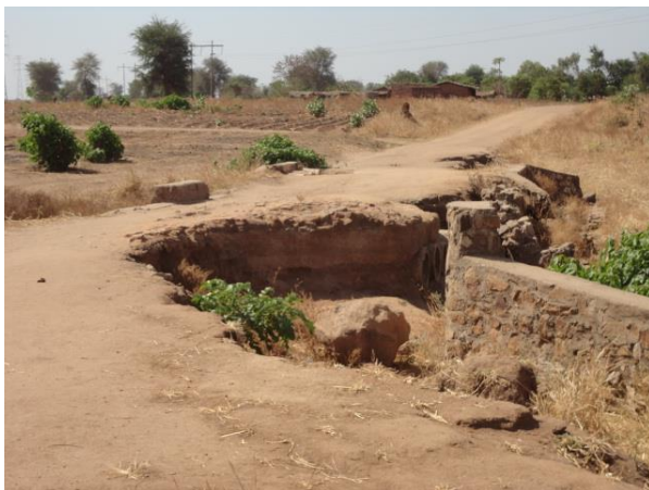
Picture 5: Erosion around existing drift
