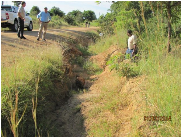
Picture 11: Typical severe erosion in RHS side drain.
