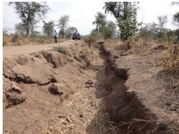
Picture 6: Severe erosion in side drain
