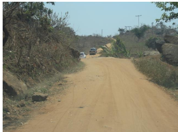
Picture 10: Section with blind curves and sharp crest that needs fully engineered solution
