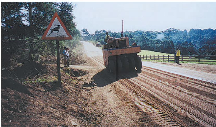
Figure 15-5: Extensive rolling of an Otta Seal- essential to achieve a good result
