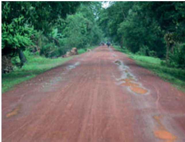
Figure.16-6: Gravel road option (Lower construction costs, higher maintenance and road user costs)
