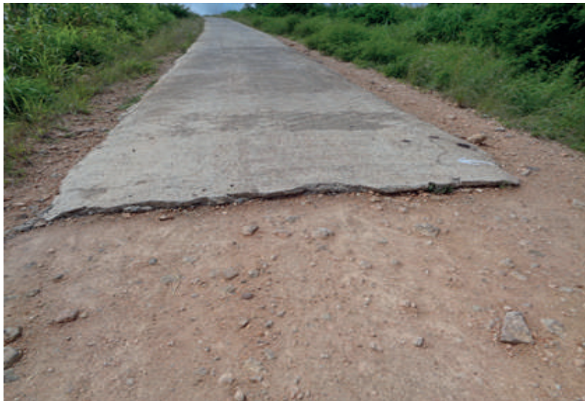
Figure 15-10: Example of two different adjoining surfacings with dangerous edge drop
