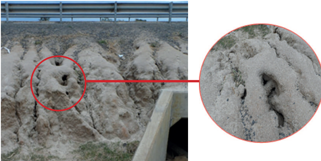
Figure 6-7: Dispersive soil showing formation of “pipes”
