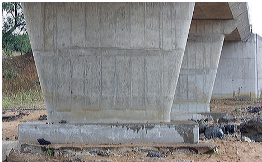
Figure 6-14: Scour at base of bridge pier foundation
