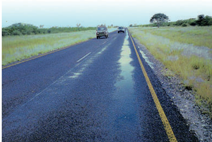
Figure 6-11: Typical manifestation of collapsible subgrade
