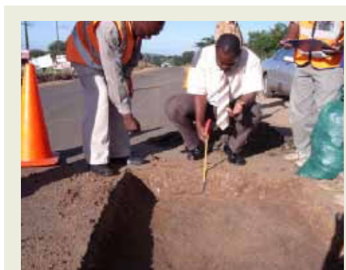
Research carried out in Malawi has provided a sound basis for understanding how LVSRs deteriorate, leading to the development of revised, standards, specifications and design methods that make better use of locally available materials.
