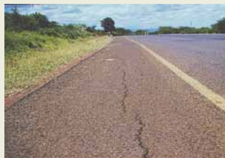
Typical longitudinal cracking and pavement deformation caused by large volumetric changes of an expansive soil subgrade.
