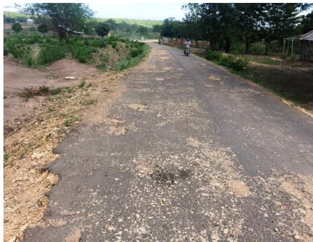
Figure 1: Sand seal section, right hand side treated with cement, left hand side treated with lime
