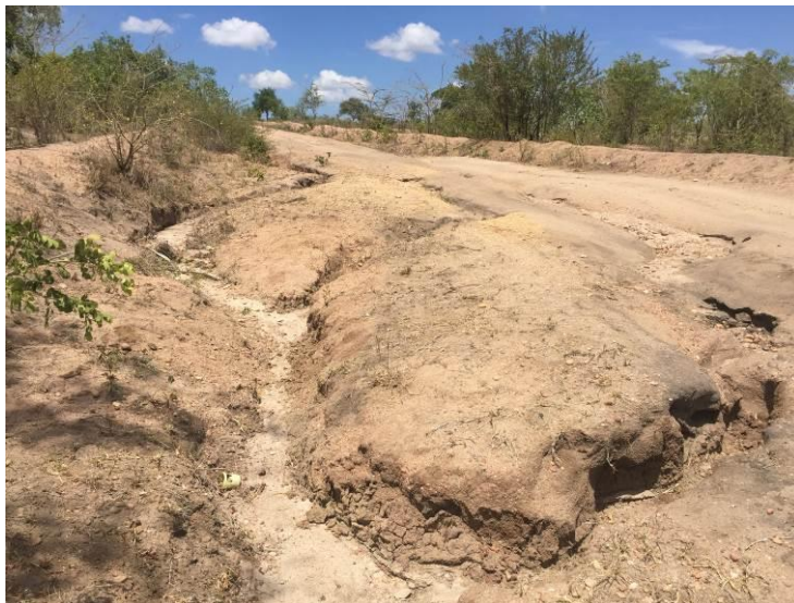
Photo A4: Severely eroded engineered natural gravel
