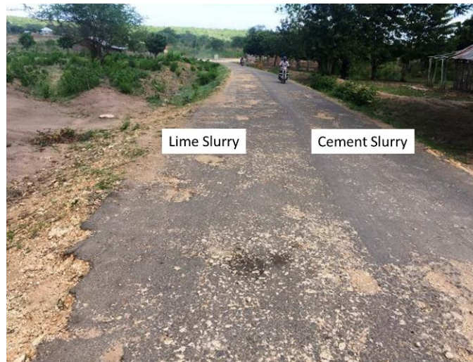
Photo A1: Slurry seal section performance
