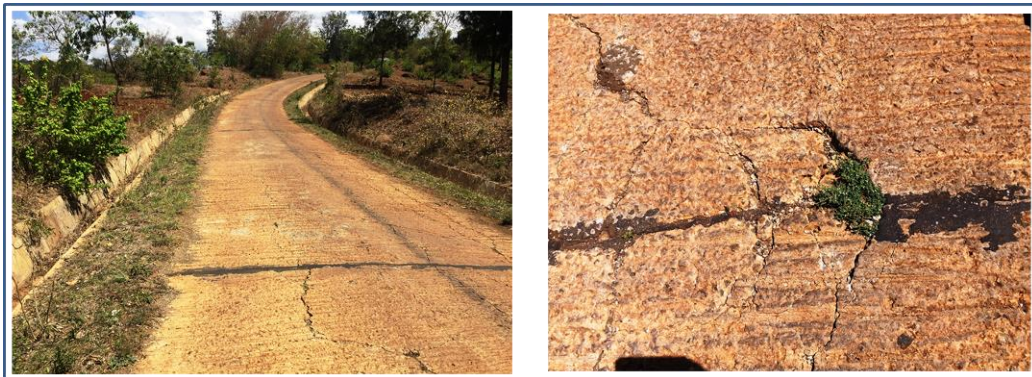
Photo A8: Defects on Unreinforced Concrete Slab section
