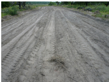
Roadbed with poor material
