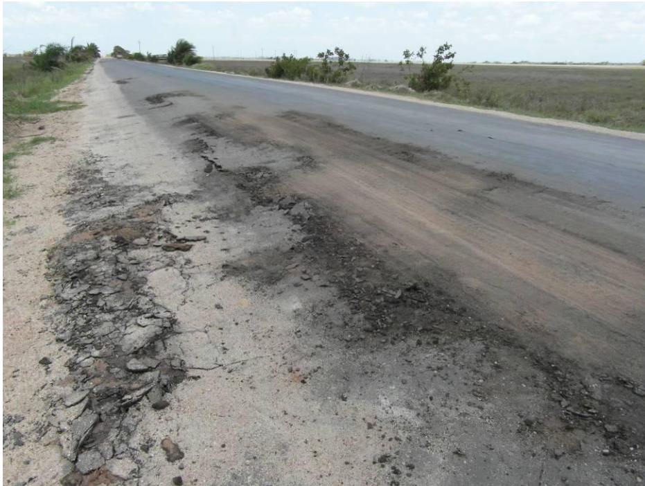
Damage on Beira Savane Road caused by heavy tipper trucks
