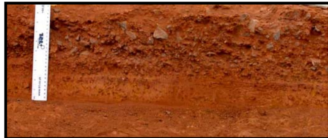
Plate 1 Laterite gravel blended with graded crushed stone as base overlying unblended laterite sub-base
