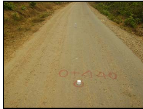
Figure 4.1 Defects in Otta Seal – possibly construction related
