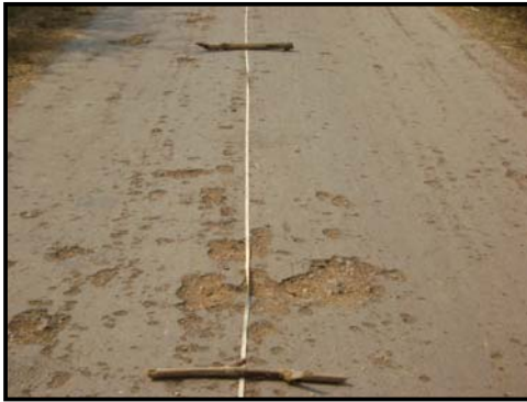
Figure 4.1 Seal erosion and shallow potholes. Road 1032.01
