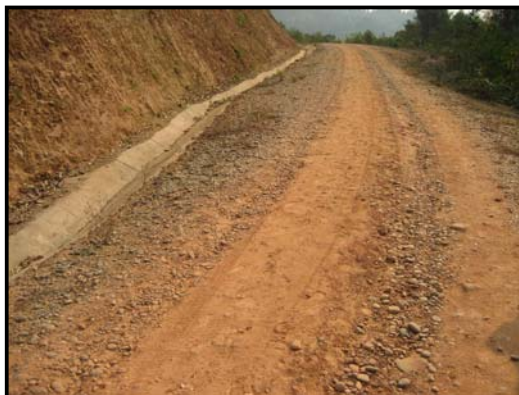
Figure 5.3 Eroded gravel on steep section of NEC package II road 201. Shape prevents run-off into well constructed drain
