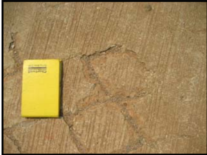
Figure 4.5 Erosion adjacent to cell boundaries
