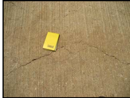
Figure 4.6 Cracks in surface screed following cell boundaries
